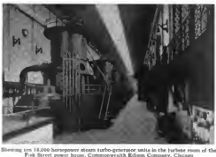
Showing ten 10,000-horsepower steam turbo-generator units in the turbine room of the Fisk Street power house, Commonwealth Edison Company, Chicago.
