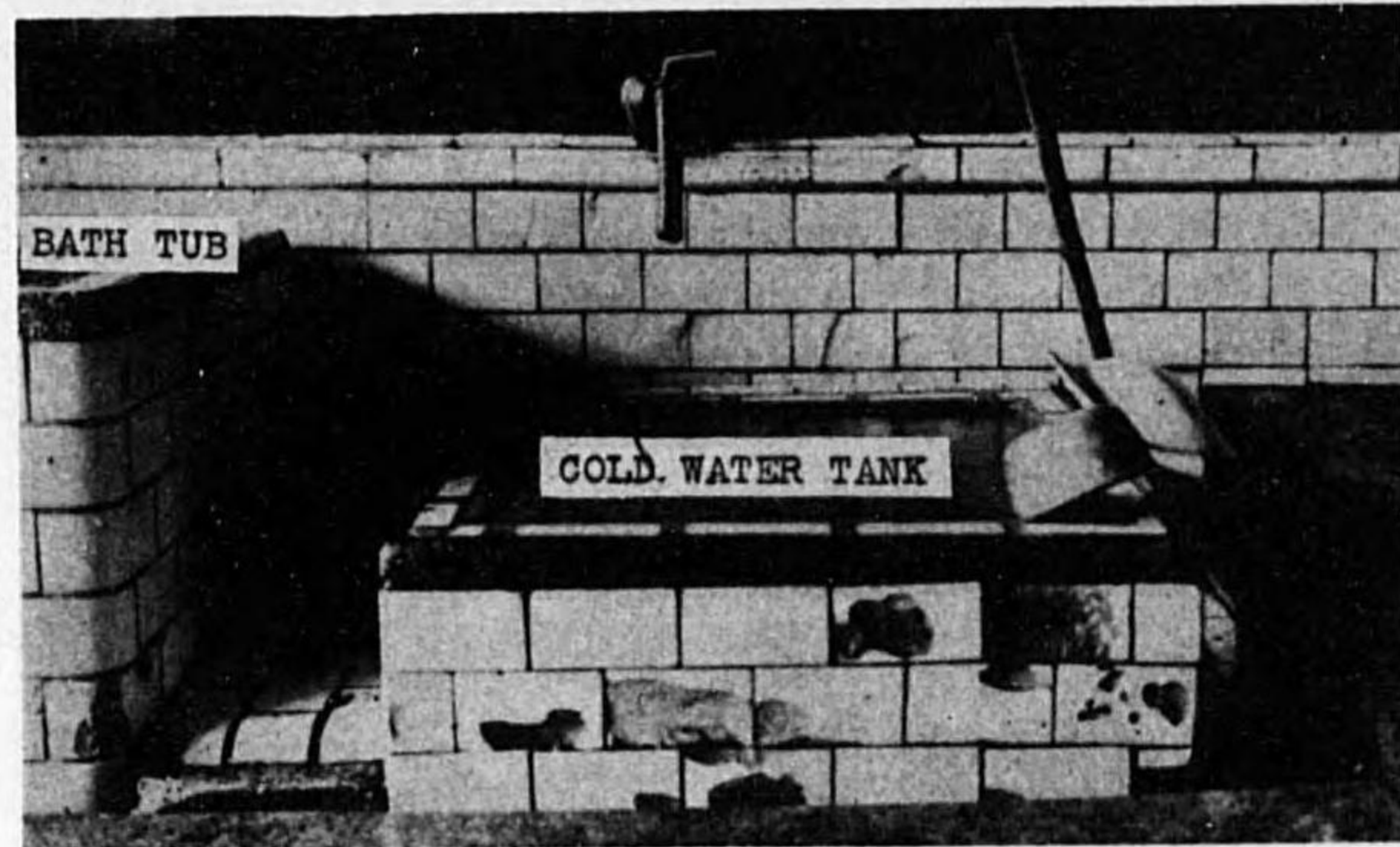
Fig. 4. Frost damaged tiles on a wall in a bath room of a hotel in Nikko.
