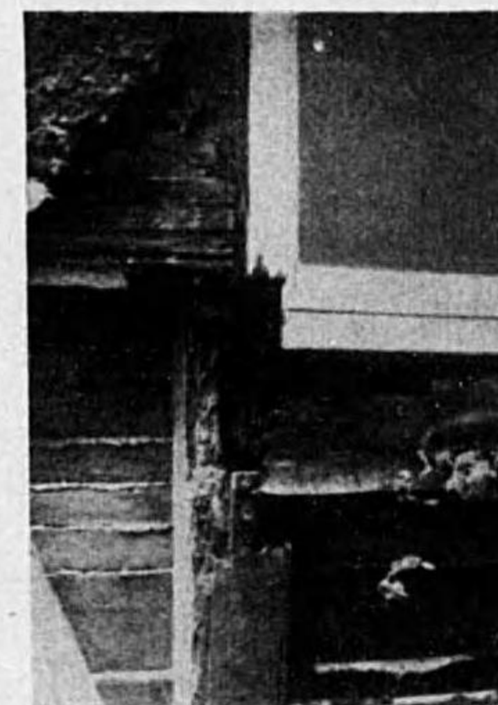
Fig. 2. Decay of wood frames of a villa.
