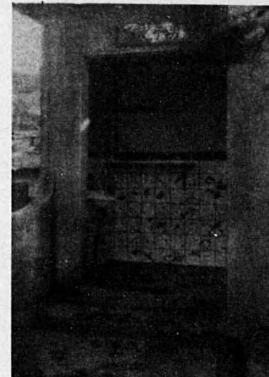
Fig. 6. Frost damaged wall tiles at a place devoid of protection.
