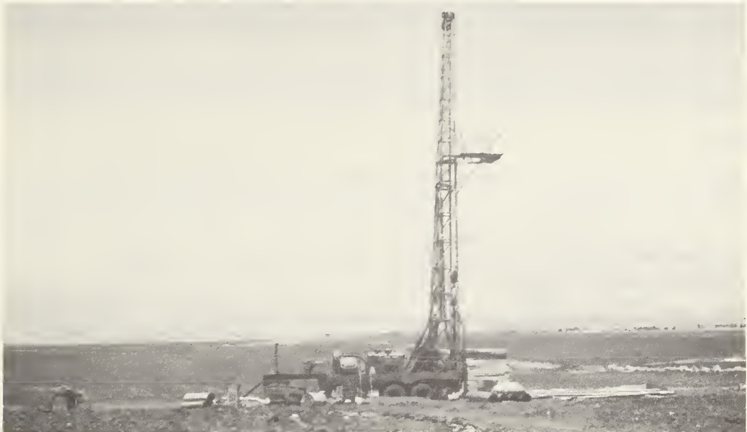
Figure 5.--Deep-well drilling in the Bekaa Valley. Irrigation is an important part of Lebanon's agriculture.
