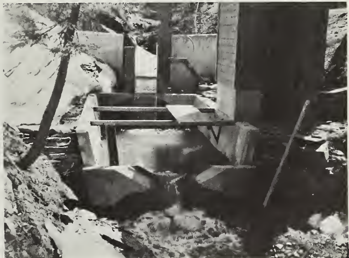
Figure 5.—Stream gaging station, Sturgis watershed 1, low discharge spring snow-melt runoff. The 120° V-notch weir carried 4.43 cubic feet per second (c.f.s.) at full head. Design discharge (25-year) is 45 c.f.s. The San Dimas flume will carry 53 c.f.s.
