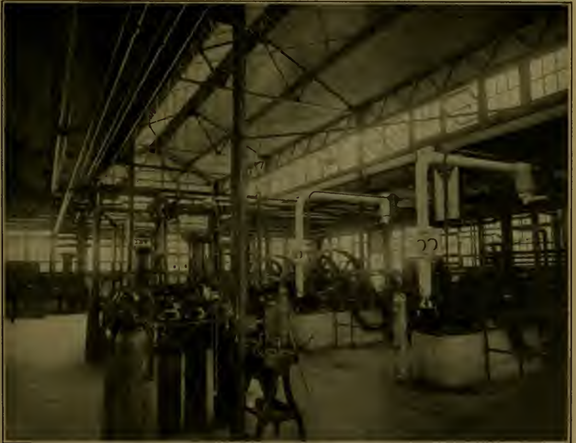
FIG. 2.—Experimental plant No. 1 (Linde system) built and used during the war. Inside a compressor building.
