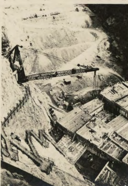
Derrick for handling concrete from low level plant
