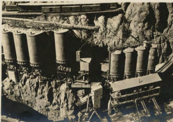
Blending, cement screening, and Hi-Mix Concrete Plants
