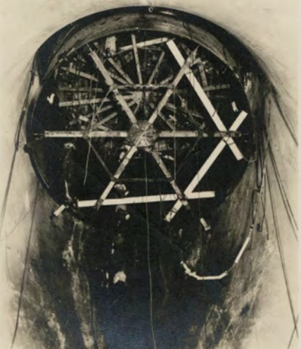
30 foot Pipe in raise No. 5
