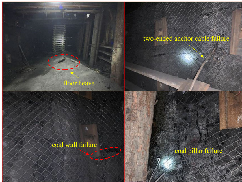
Figure 2. Roadway deformation and failure.
