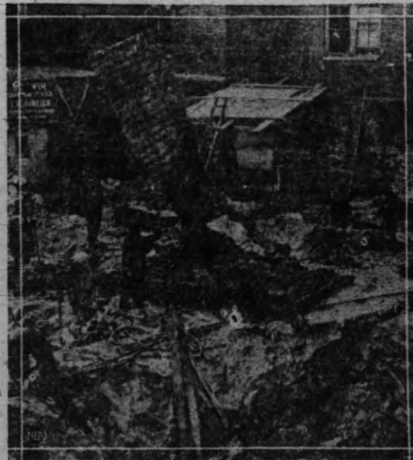
OVERCOMING DIFFICULTY—Excavating in the solid granite of Manhattan for the giant skyscrapers of New York is a task. Dynamite is about the only pyrotechnic method giving quick results. Yet in the crowded streets surrounding the work lie many chances of fatal accident from the flying debris. To obviate this, steel blankets are spread over the ground underneath which the charge is planted. Photo shows these blankets being put in place.
