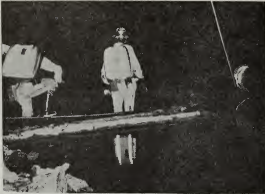
Figure 2-4-4. Inspection of Separator Room Team wearing oxygen breathing apparatus found separator room in good condition. Clear water behind sediment dam shows in foreground. Looking NW
