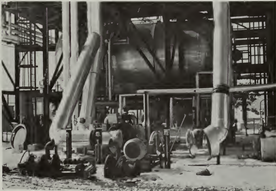
Figure 3-1-3. Streamlined Piping for the C-102 Auxilliary Suction Blowers.
