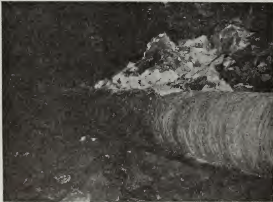
Figure 2-4-5. Caving of Retort Zero Entry Inspection team found entry to Retort Zero caved out to junction with Product Drift.
