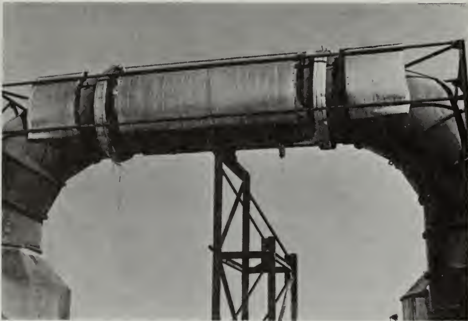
Figure 3-1-7. Expansion Joints Between the Incinerator and the Scrubber
