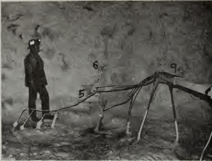
Figure 3-1-9. Instrumentation Station Note drill casings in floor and thermocouple leads to cable tray in right foreground. Shot Crete and Miracoat sealant were applied to help limit leakage.
