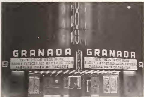
New attraction display panels and letters installed on the marquee of the Granada theatre in Dallas. The equipment, by Wagner, was installed by the Modern Theatre Equipment Company. Letters are colored plastic.
