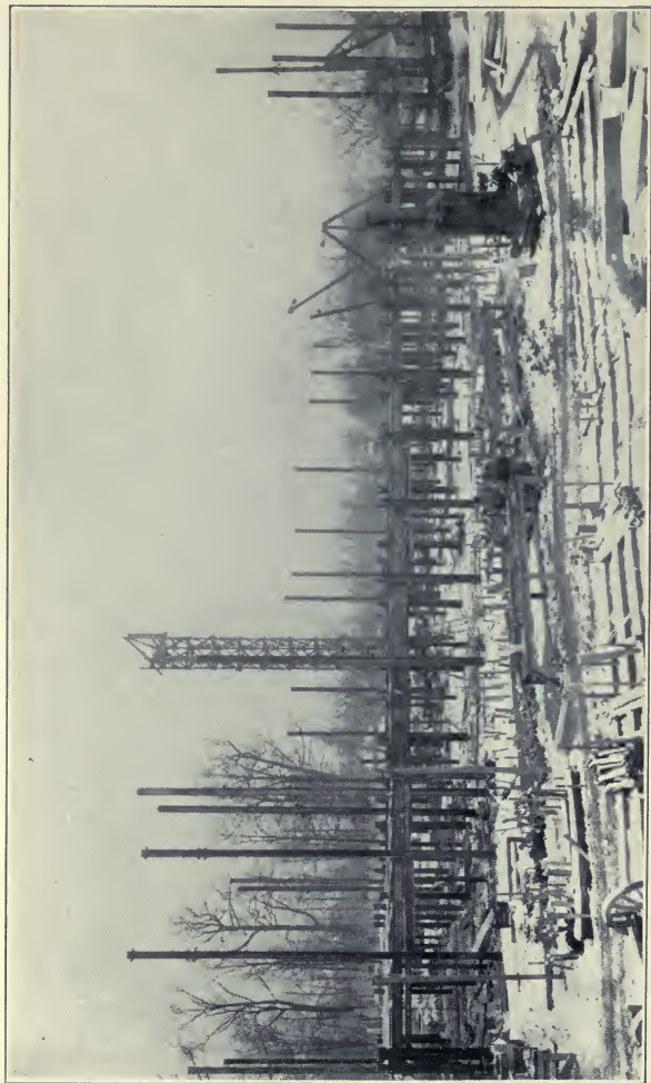
Art Museum after seven and one-half months' work, December 29, 1913. Foundation is finished; framework is started
