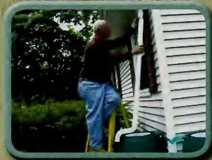
Extension program participant installing a rain barrel at his home after the program.
