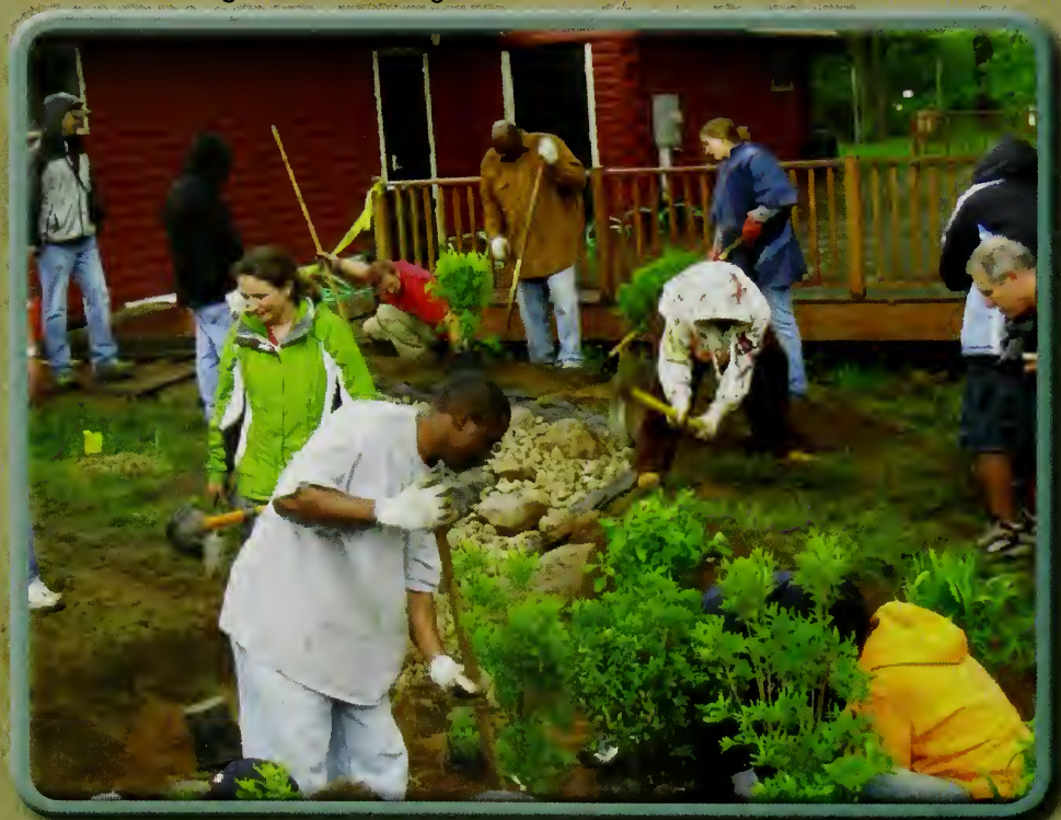
Small contractors get hands-on training in the construction of "rain garden" vegetated stormwater practices.
