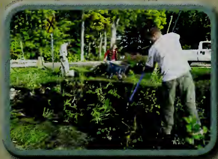
University of New Hampshire and Rutgers University collaborative programming installed this rain garden in Portsmouth, NH.
