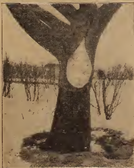
The Cavity in the Trunk of This Tree Has Been Filled With Cement
