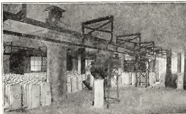
These automatic scales are movable and may be connected with any of our seed storage bins on floor above.
