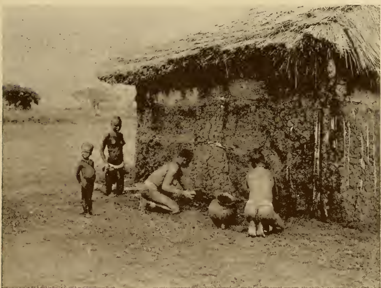
FIG. 38.—Women of Liri on the Albert Nile repairing the wall of a hut with mud. The walls are made with wooden supports and between these are placed rows of stalks of elephant grass partly buried in the ground and fastened together with grass. The whole is then covered with mud and a roof built so that it overhangs and protects the walls from the erosive effect of rain.
