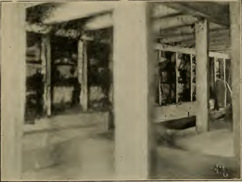
INTERIOR OF STABLE, SHOWING MANURE ON WALLS.
