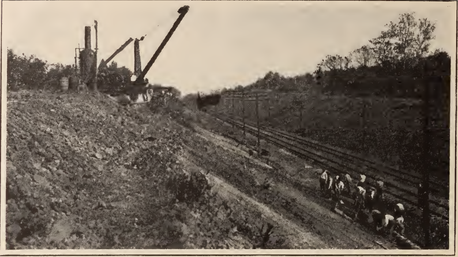
No. 2—SPECIALLY CONSTRUCTED CONTAINER LOADED WITH DIRT, BEING HOISTED TO THE TOP OF THIS CUT
