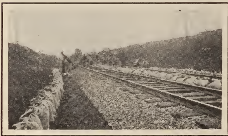
ARRANGEMENT OF SACKS TO FACILITATE LOADING OF DIRT ON WORK TRAINS OR TRUCKS
