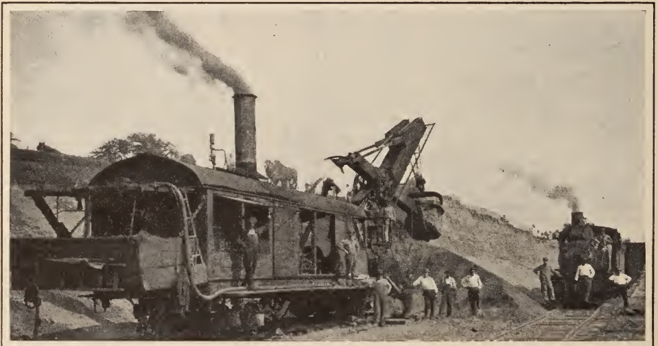
CRANE ENGINEER GEORGE FLANNIGAN, YARD FOREMAN ALBERT GROMBAUGH AND CREW LOADING BALLAST AT CINCINNATI, HAMILTON & DAYTON PIT AT HAMILTON, O.
