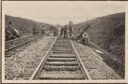
TRACK DRESSED, LEAVING OPEN CRIBS BETWEEN RAILS FOR DISTRIBUTION OF BALLAST FROM ROGER CARS
