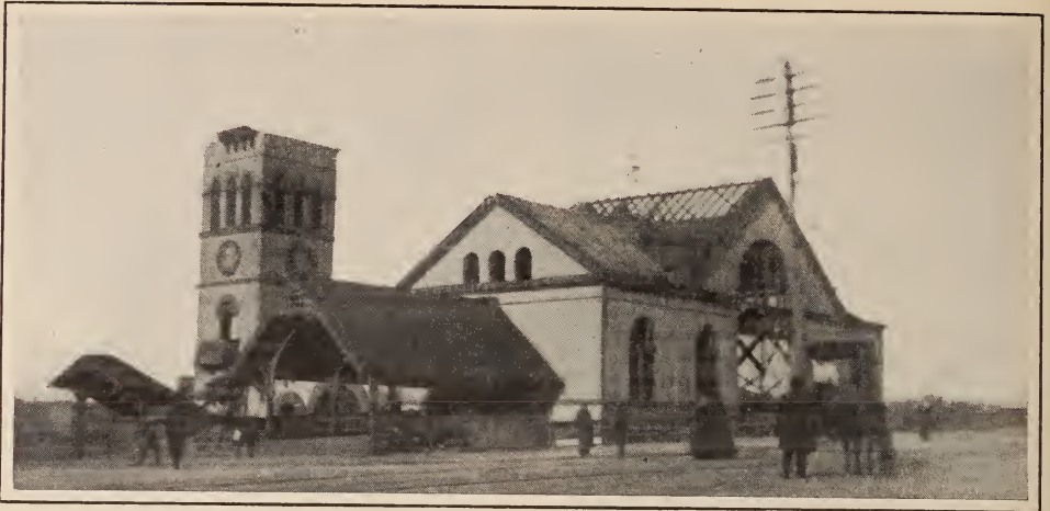
OLD COMPANY STATION IN WASHINGTON, D. C., IN PROCESS OF DEMOLITION FEBRUARY 5 TO MARCH 15, 1908
