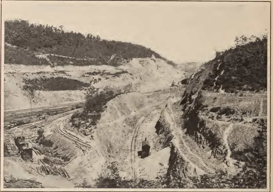
APPROACH CUT OF RANDOLPH TUNNEL IN FOREGROUND AND DOE GULLY CUT IN PROCESS OF EXCAVATION IN BACKGROUND
