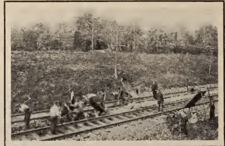
ARRANGEMENT OF FORCES WORKING SCREENS THROUGH CUT, SHOWING THE PROCESS OF SACKING DIRT
