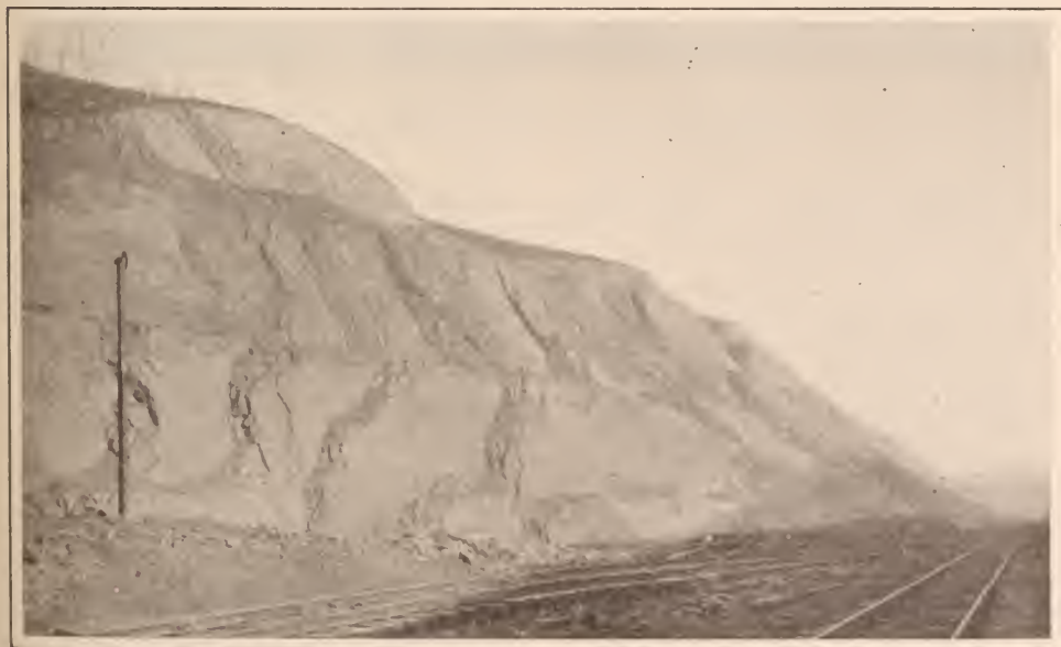
DOE GULLY CUT, CLEARLY SHOWING THE BENCHING OF ROCK CLIFFS TO PREVENT SLIDES
