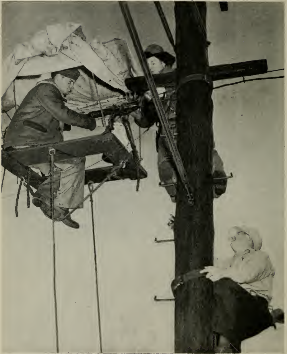
TWO MARINE CORPS STUDENTS make a practice repair on a plant school telephone cable as an operating company instructor supervises their work. See "Bell System Schooling for Service Men," beginning on page 215
