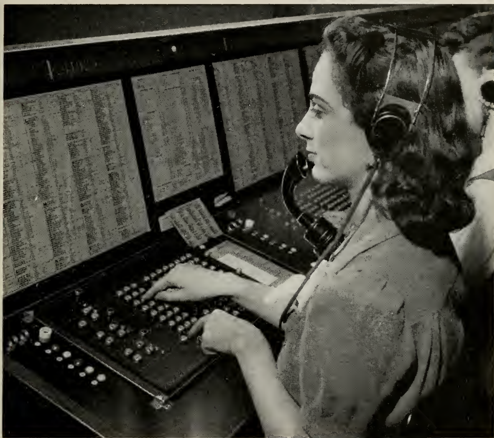
OPERATORS AT the No. 4 toll switchboard in Philadelphia handle inward and through calls. The keys which they press set up electrical impulses just as do the dials which subscribers use to make local calls
