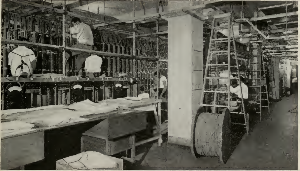
INSTALLING THE world's largest private branch switchboard in the War Department. Installers worked around the clock to speed it to completion
