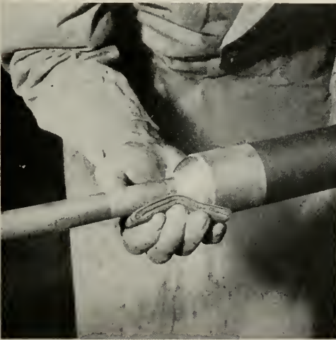
IT TAKES a skilled craftsman to wipe a joint in a cable
