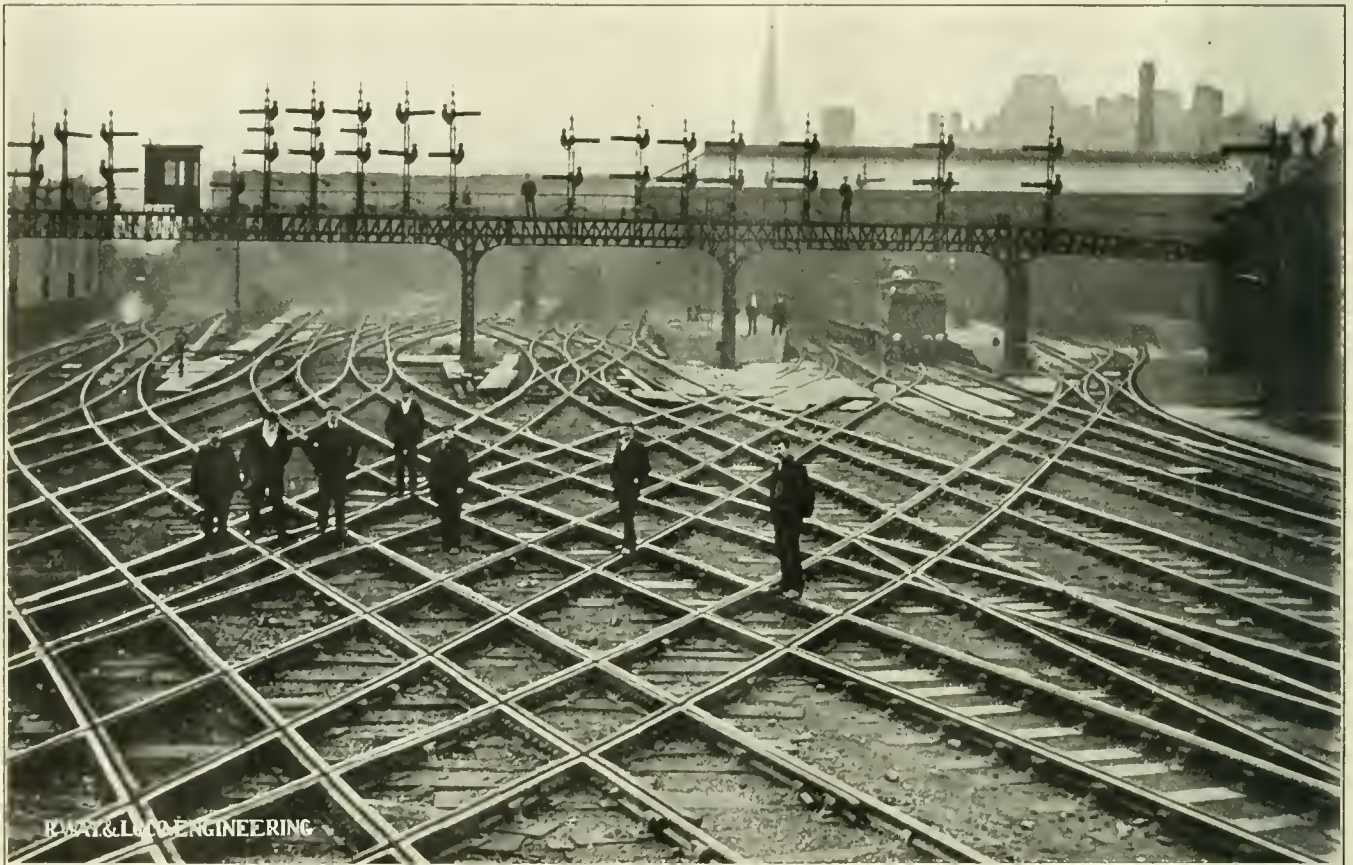
INTERLOCKING PLANT, NEWCASTLE CENTRAL STATION.
