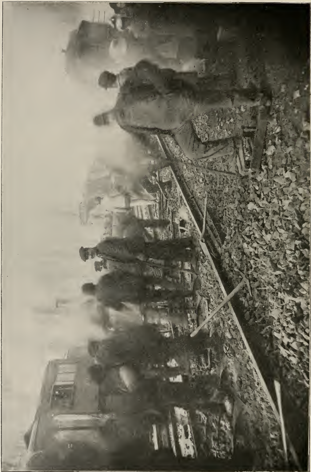
THE WRECK OF THE PENNSYLVANIA FLYER—STEEL TIES, TWISTED AND TORN, BEING REMOVED TO BE REPLACED WITH WOOD.
