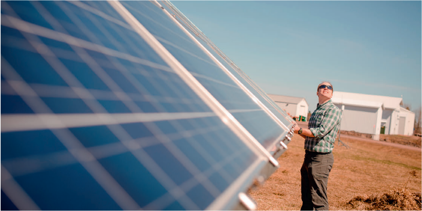
Figure 3.17 A polycrystalline PV array that powers a research center in the Midwest U.S. that is used for cold weather testing.
