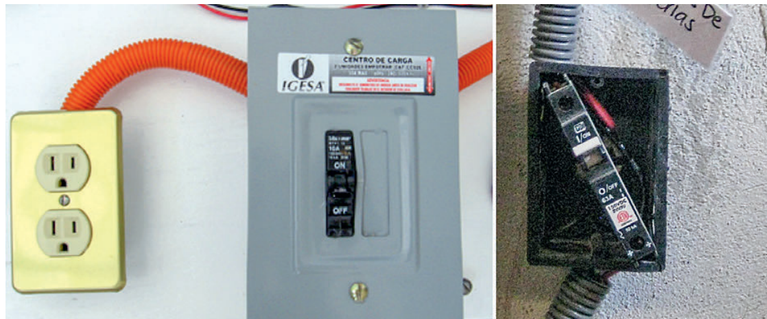
Figure 5.8 120 VAC - 10 A breaker in a breaker panel with conduit and 120 VAC plugs (left) and a 150 VDC - 63 A breaker in a makeshift housing from a junction box (right). appropedia.org/UTC_photovoltaic_learning_station appropedia.org/Practivistas_solar_2015
