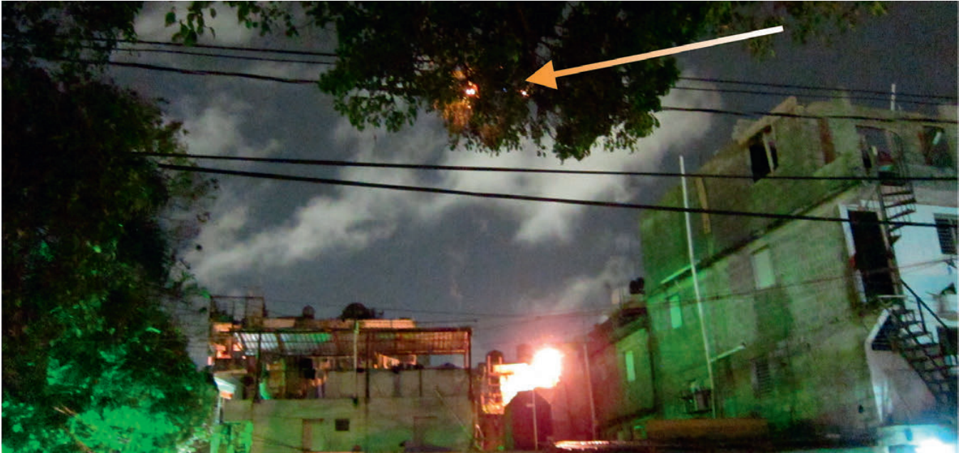
Figure 2.2 Electrical lines on fire in La Yuca.
