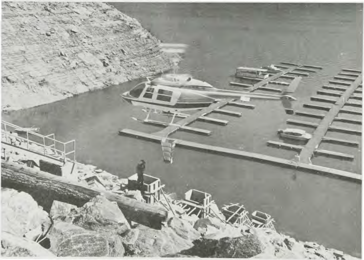
HELICOPTER CARRYING CONCRETE FOR STAIRWAY STEP EXPANSION AT BIG EDDY BOAT MOORAGE AREA DWORSHAK RESERVOIR, 1978
