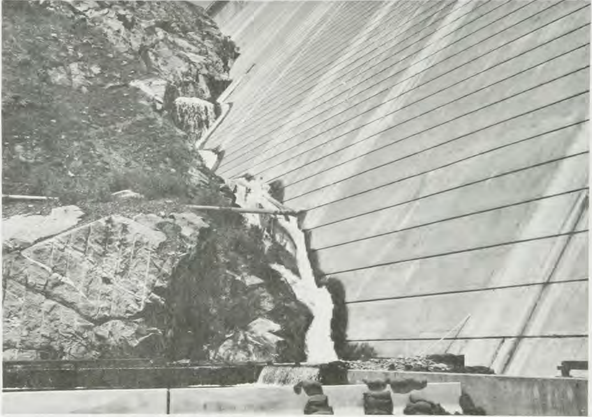
THE CRACK AT DWORSHAK DAM
