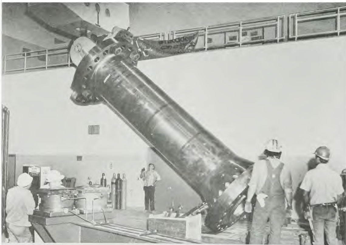
LOWERING THE UNIT 6 INTERMEDIATE TURBINE SHAFT, AT THE LITTLE GOOSE DAM SECOND POWERHOUSE
