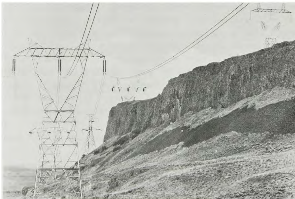
TRANSMISSION TOWERS AT LOWER MONUMENTAL DAM
