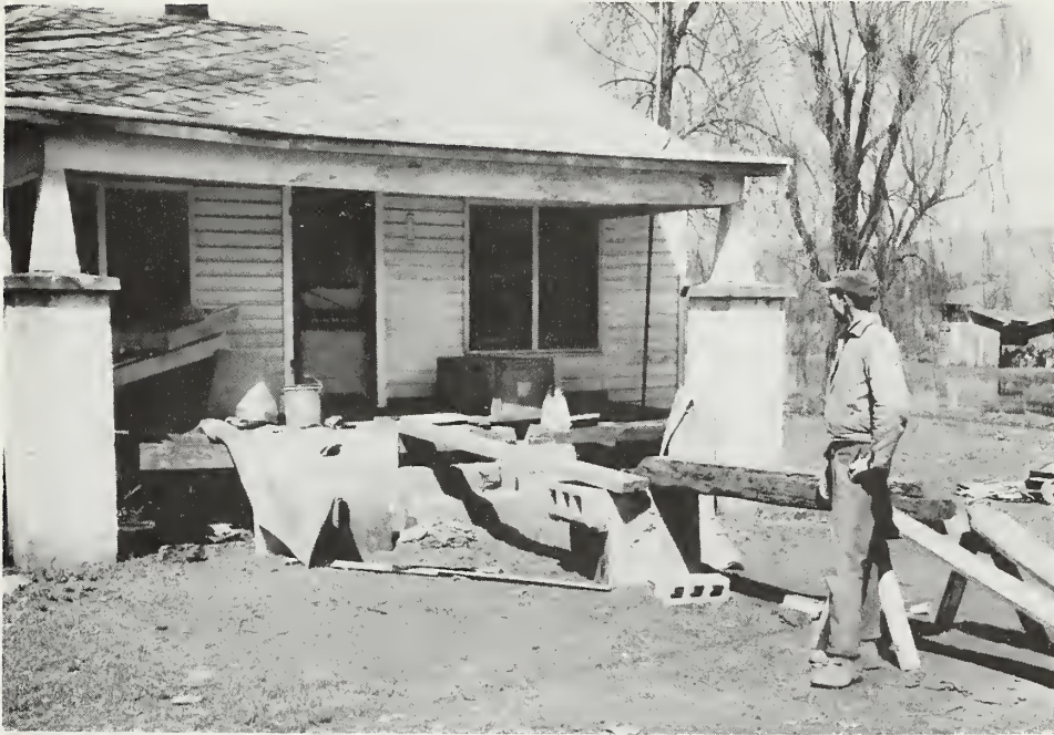
Damage to Mrs. Bill Nelms' home and furniture in city of Philadelphia. Floodwater depth inside house on March 12, 1963 was about 18 inches.
