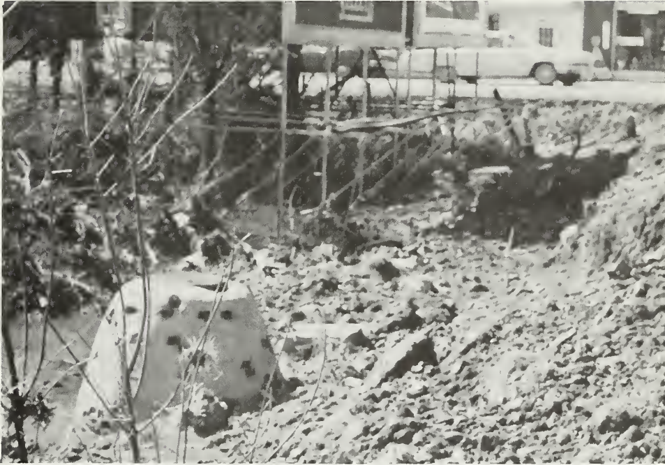
Erosion damage in main business district of Sweetwater to U. S. Highway 11.
