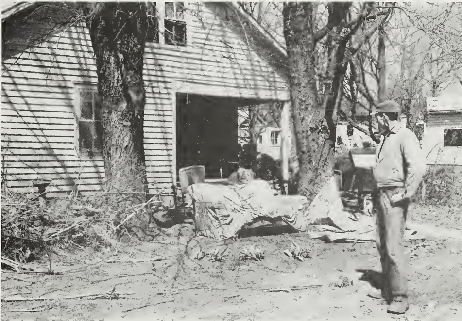
Mr. Roy Bledsoe looking at damage to Mrs. Joe Clark's home and furnishings in the city of Philadelphia. Floodwater depth inside house on March 12, 1963 was about 30 inches.
