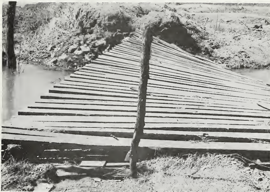
A typical scene of floodwater damage to on-farm bridges along Sweetwater Creek.
