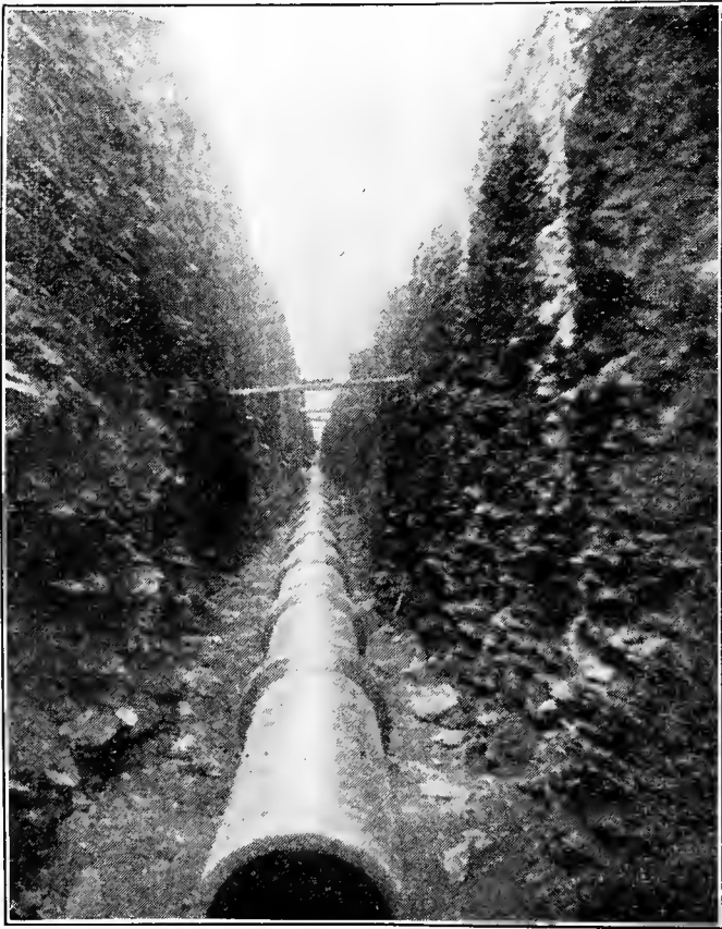
A Typical Pipe Line of a Water Carriage Sewer System --Sewer on Linwood Avenue.
