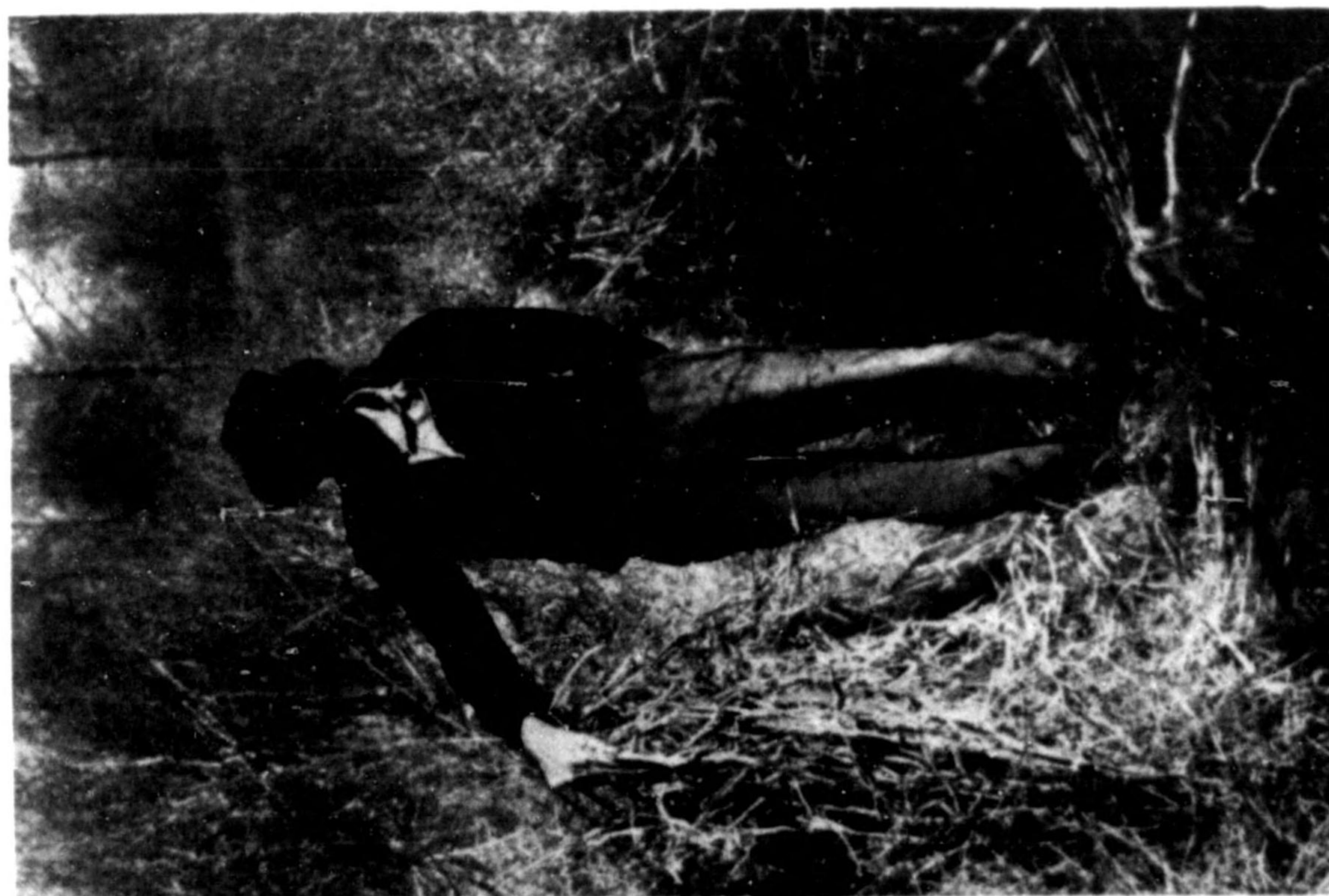
FIGURE 11.—Heavy vegetation growth between the joints of butt-joint precast slabs.
