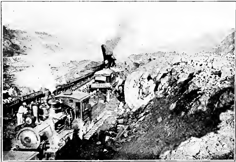
STEAM SHOVEL AT WORK ON THE SITE FOR THE PEDRO MIGUEL LOCKS.
