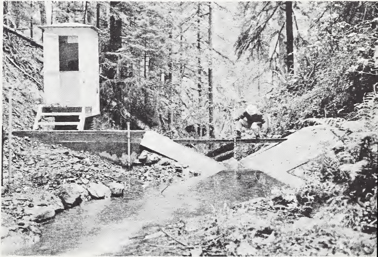
One of the trapezoidal flumes installed on the three matched drainages.
