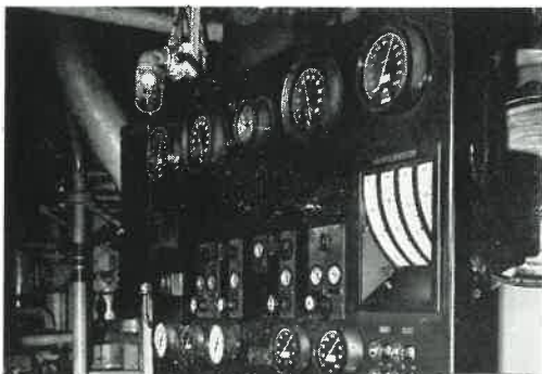
Hagan Control Panel (T-2 Tanker)
