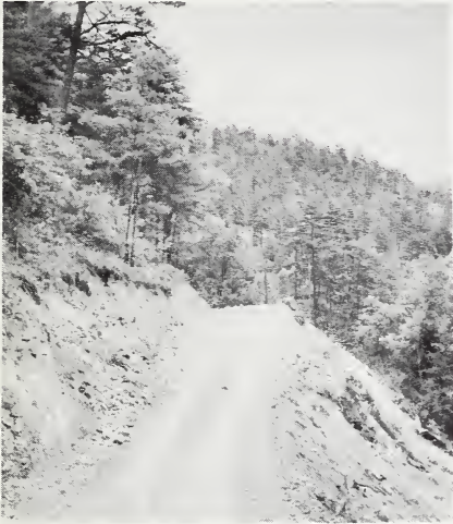
Figure 7—Completed section of road in steep terrain. Note inslope of road bed and slopes of road banks.
