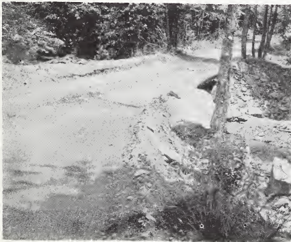
Figure 16 — Approach to temporary bridge in logging road. Note uniform grade of approaches and bridge floor.
