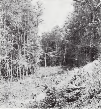
Figure 5 — Right-of-way clearing is the first step in the construction of a woods road.
