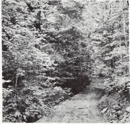
Figure 8—Clearing to inadequate widths retards drying out of road surface. This road has been in existence for a number of years. Note how crowns of trees have closed in over right-of-way. Some "day-lighting" is desirable here.
