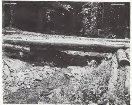
Figure 17 — Side view of same bridge. Note bridge components — log abutments, stringers, sawn timber decking, run-planks, and wheel guards.
