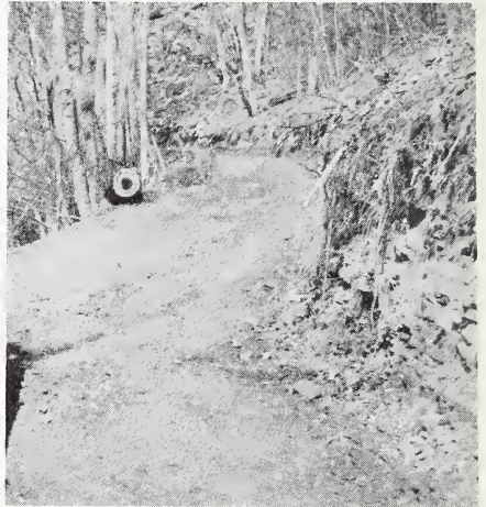
Figure 6 — Completed section of low service, low-speed timber haul road. Note steep slope of cut bank.
