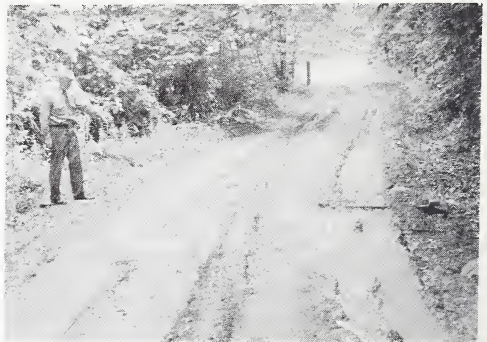
Figure 18 — Box culvert in this section of road has lost its usefulness. Too shallow side ditch and clogging of culvert resulted in heavy rutting of road. Drainage structures must be properly installed and maintained.
