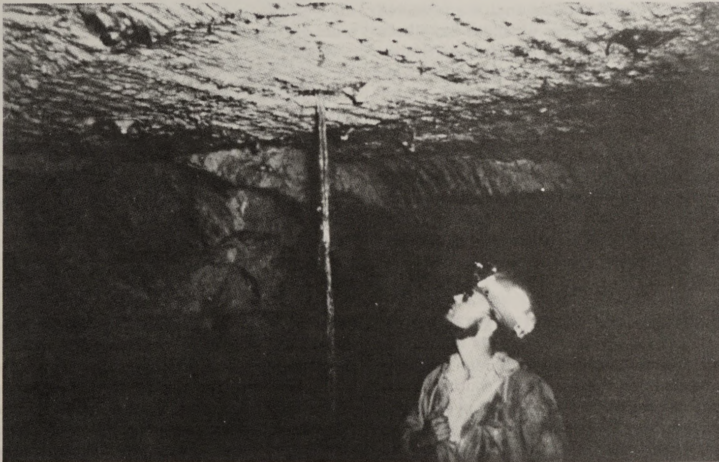
FIGURE 8.—Water draining from a bolt hole in the sandstone roof of an underground mine in Utah (from Lines and others, 1984).
