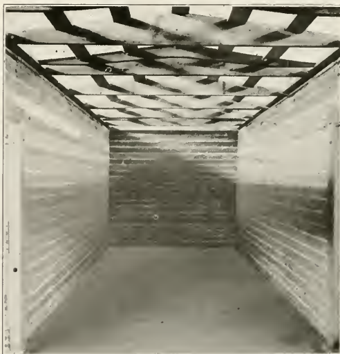
Interior of the Car after the Application of the Sub Floor and Outside Sheathing
