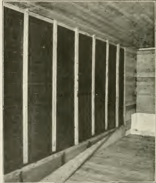
Interior of the Car Showing the Completed Side Wall Insulation and Method of Sealing the Joint at the Floor
