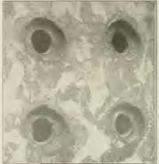
Effect of Corrosion Around Staybolts
