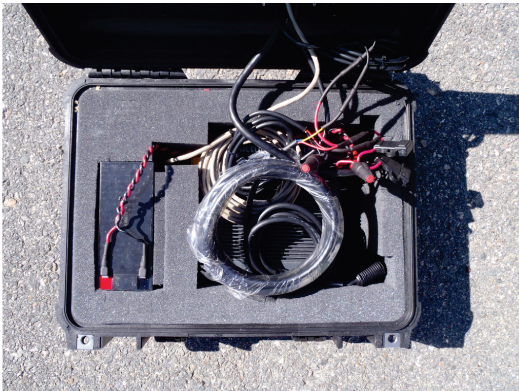
Figure A2. LSS-2, 12-V power source and wiring.
