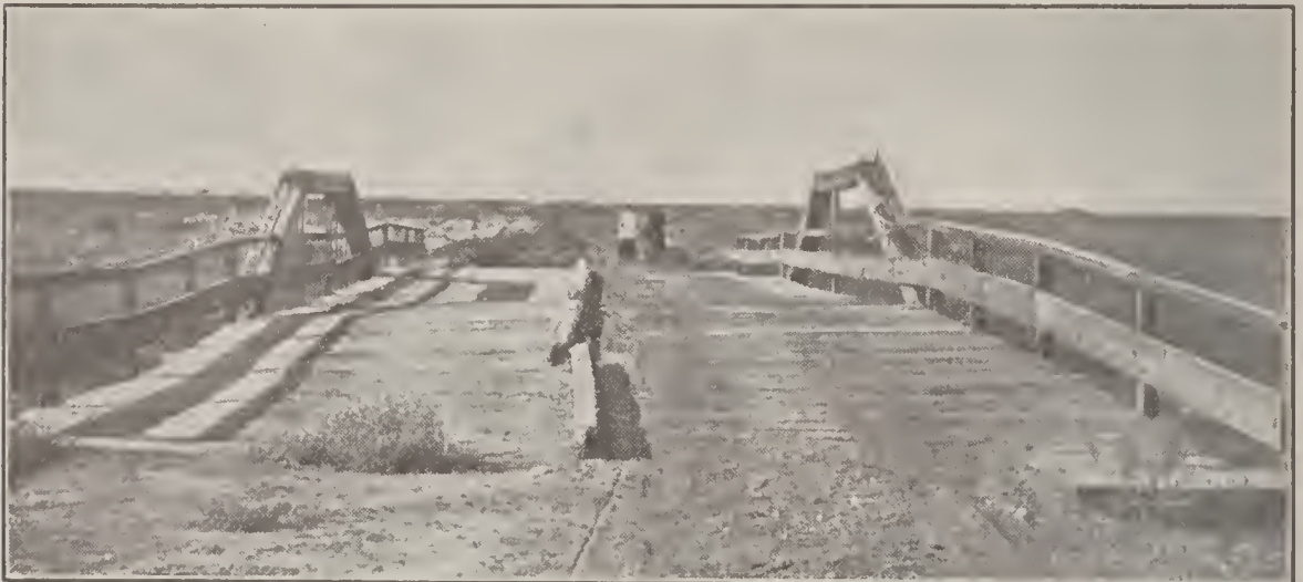
Dangerous Wooden Bridge
