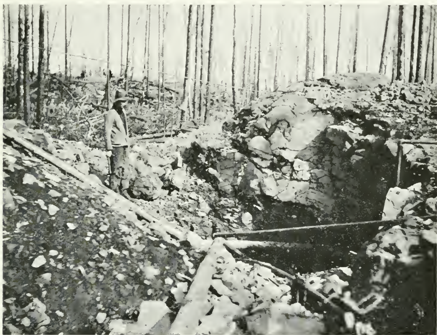
Fig. 34—Entrance to inclined shaft, Howey-Cochénour-Willans gold prospect, Lightning river area, Holloway township.
