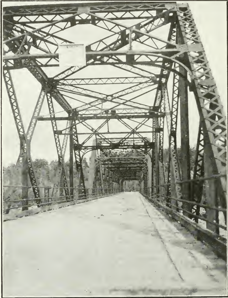
The Interprovincial Bridge crossing the Ottawa River at the Joachim Rapids, near the Trunk Road from Pembroke to Mattawa.
