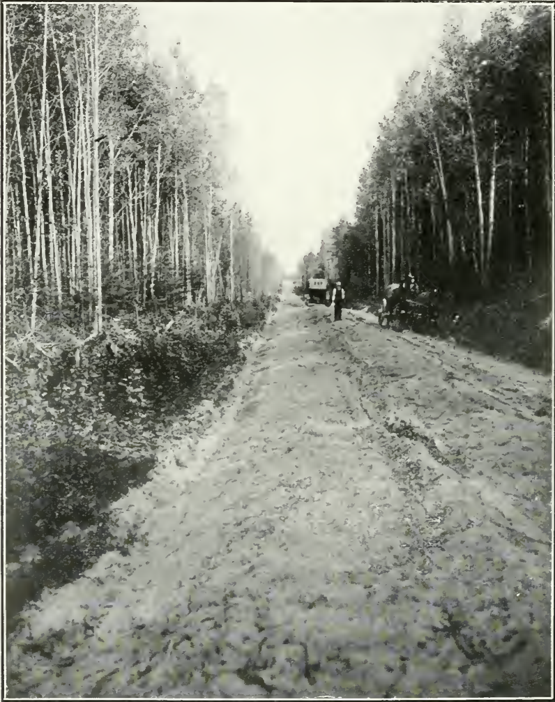
A typical view of a road cut out and newly graded through the virgin forest; near Wabigoon, District of Kenora.
