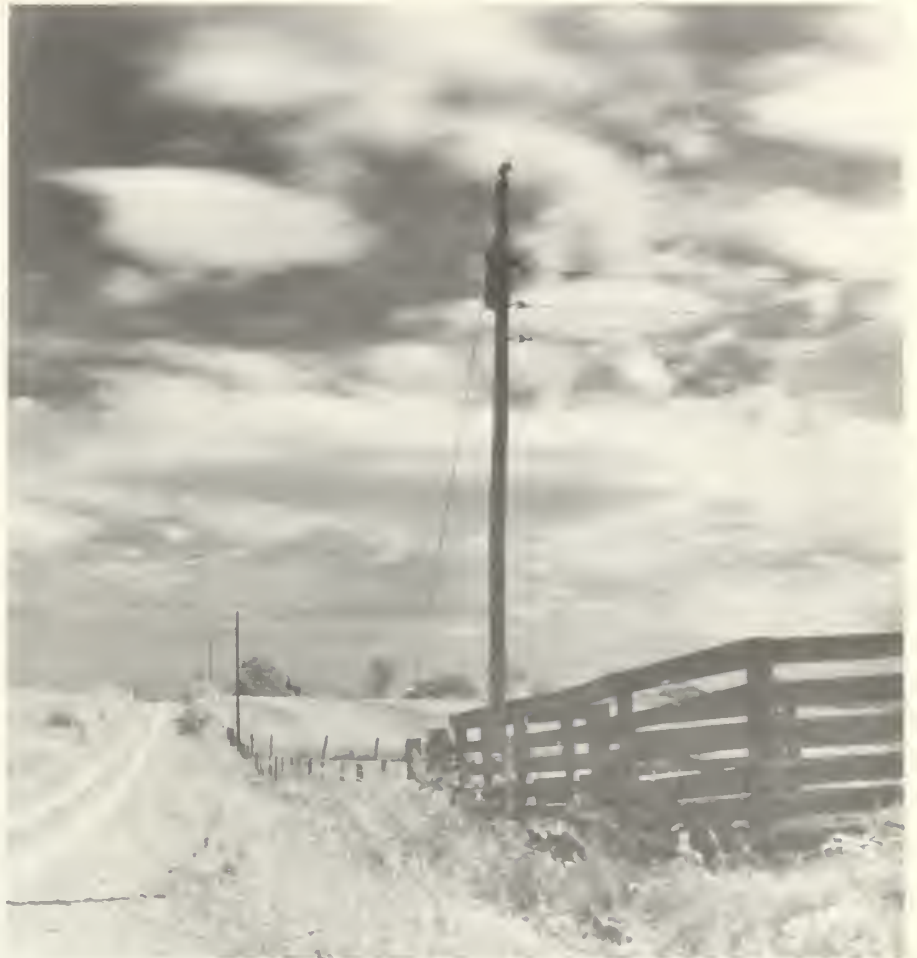
Simple but sturdy construction, pioneered by REA, kept costs down, while maintaining reliability.
