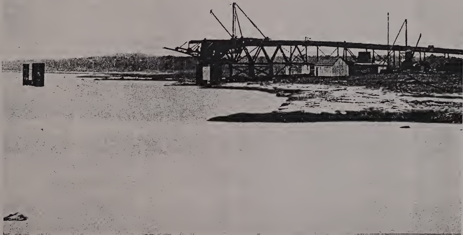
The Partly Completed Highway Bridge that will Span the Canal between Buzzards Bay and Bourne, Feb. 1911.
