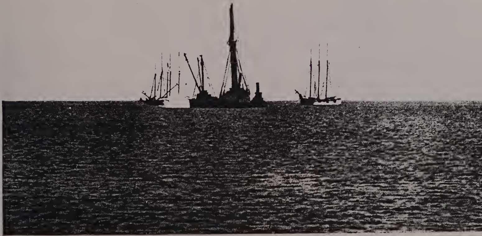
Beginning the Construction of the Breakwater. The First Load of Granite for the Great Seawall, June 1909.
