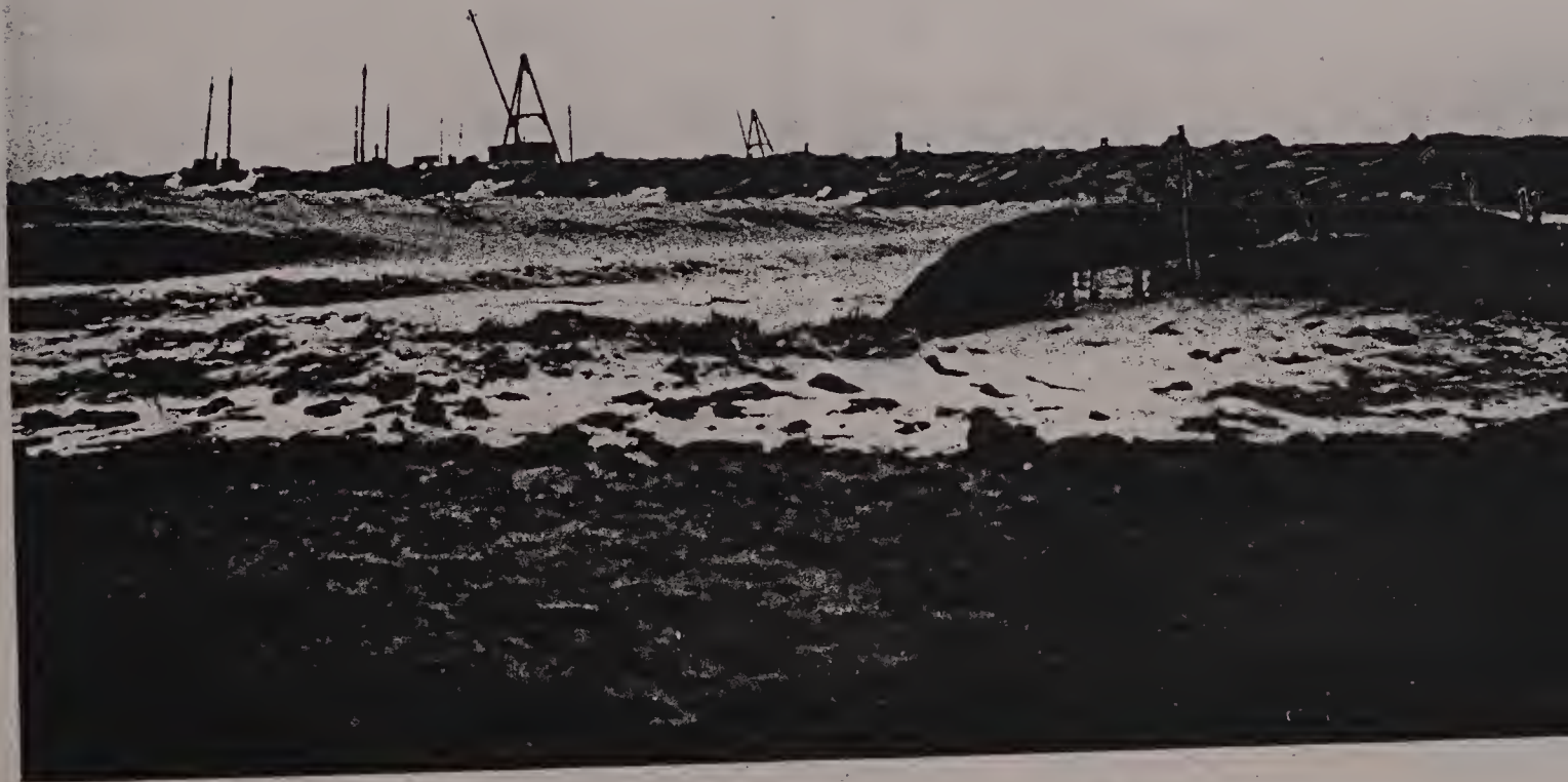
Working on Breakwater, Sept. 14, 1910. * Discharge Pipe from Dredge, Sending "Spoil" Over Breakwater.
