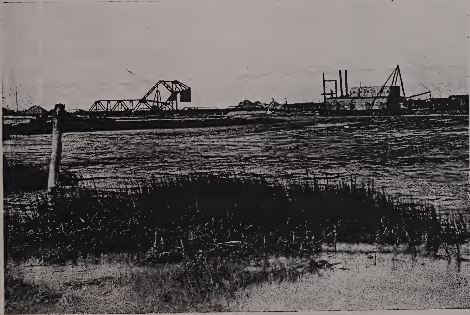
Completed Roll Lift Railroad Bridge Spanning the Canal and Dredge on Buzzards Bay End of the Waterway Nov. 1910
