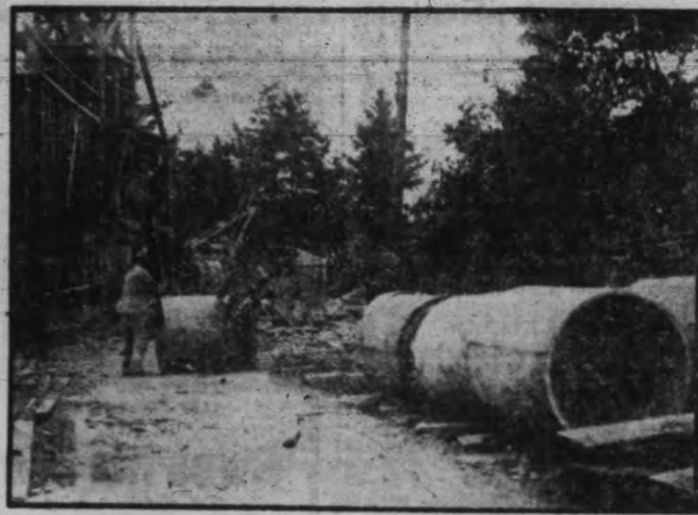
The above picture shows the character of the pipe used in the Northwest sewer tunnels, now rapidly approaching completion.
