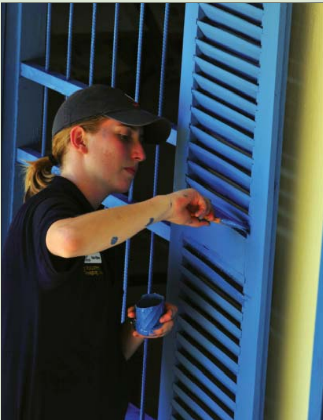
SIHANOUKVILLE, Cambodia - Kate Villars, a San Diego Pre-Dental Society volunteer from the University of California embarked aboard the Military Sealift Command hospital ship USNS Mercy (T-AH 19), paints window shutters at the Andaung Thma School during a Pacific Partnership 2010 engineering community service event. Mercy is in Cambodia supporting Pacific Partnership, the fifth in a series of annual U.S. Pacific Fleet humanitarian and civic assistance endeavors to strengthen regional partnerships. (U.S. Army photo by Sgt. Craig Anderson/Released)
