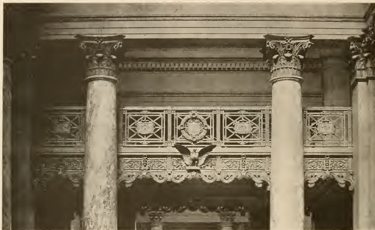
CAST-IRON RAILING AND FACIA THIRD FLOOR CORRIDOR Minnesota State Capitol Building, St. Paul, Minn. Cass Gilbert, Architect
