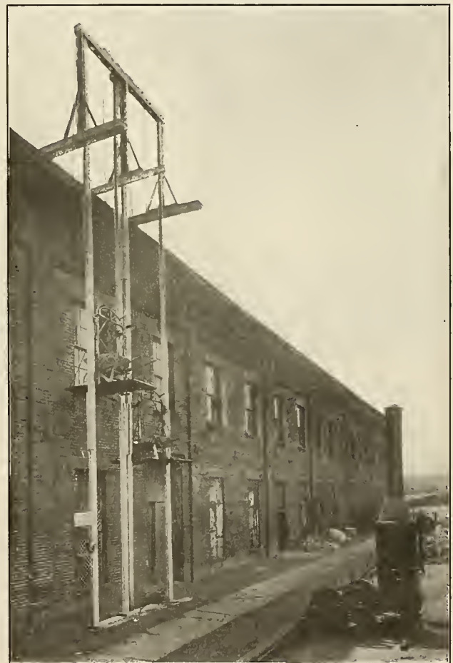
FIG. 3. VIEW OF METHOD EMPLOYED To install a Double Acting Elevator on the Outside of a Building for Repair Work
