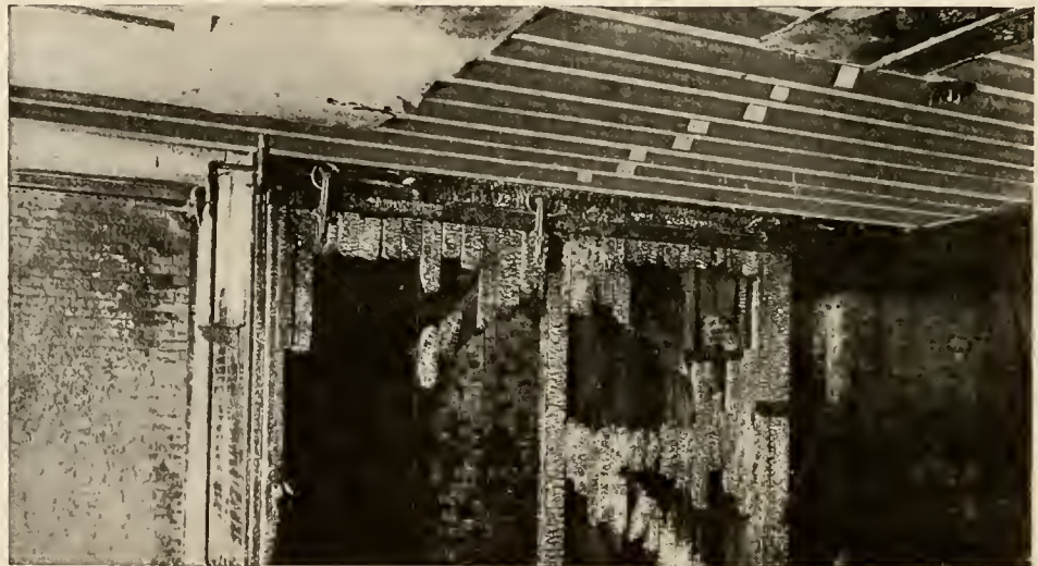
FIG. 1. SECTION OF A BUSINESS BUILDING SHOWING CONDITION OF BEAMS WHEN PLASTER BOARDS WERE TORN DOWN BY FIREMEN AFTER A FIRE
