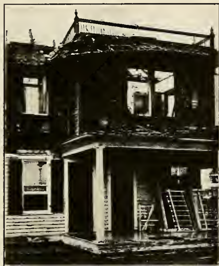
FIG. 2. COTTAGE SHOWING WHERE THE CLAPBOARDS WERE BURNED AWAY
