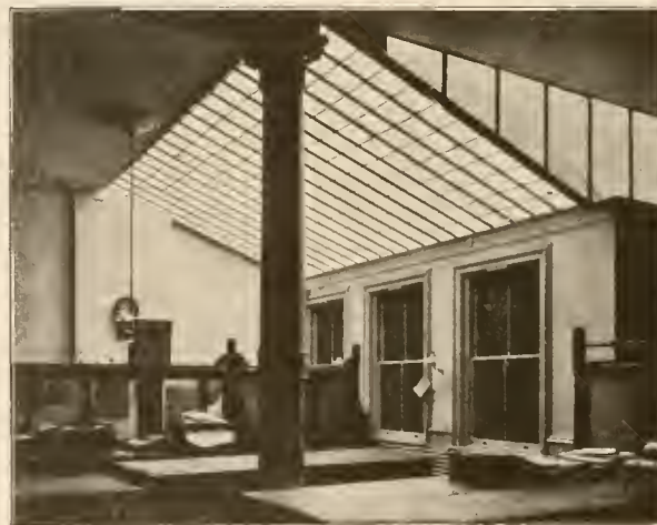
FIG. 8. THE SKYLIGHT PRISM THAT CAN BE MADE AND KEPT TIGHT WITHOUT REPAIRS
