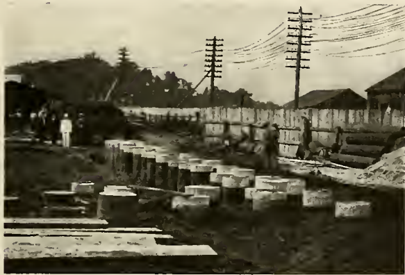
FIG. 5. RAYMOND CONCRETE PILE Used in the Construction of the Academic Building, Annapolis, Md.
