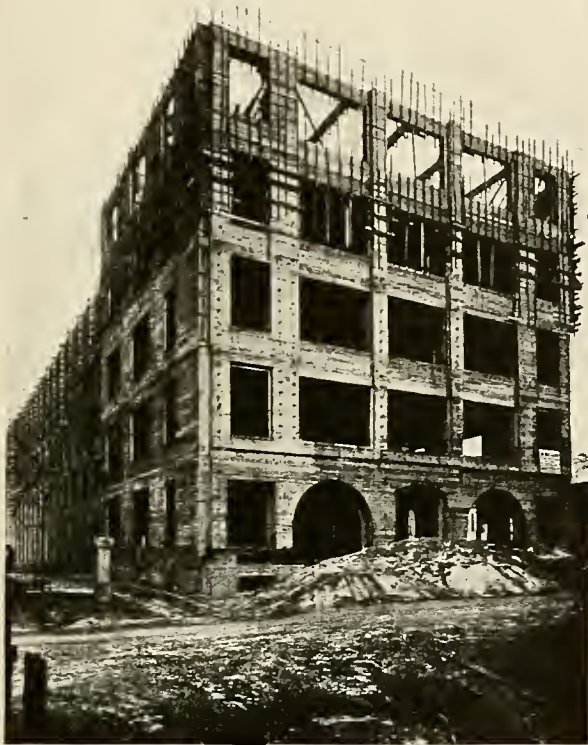
PUGH POWER PLANT, CINCINNATI Ditoe & Wisenall, Architects. Solid Concrete. Whitehall Portland Cement used.
