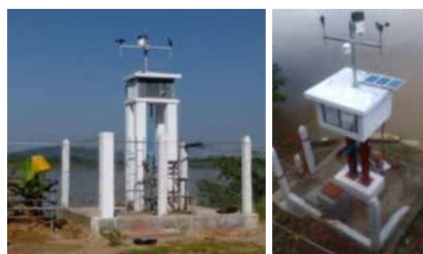
Figure 6.8.1. Hydrometry Monitoring Systems. Photo ©IHP Myanmar
