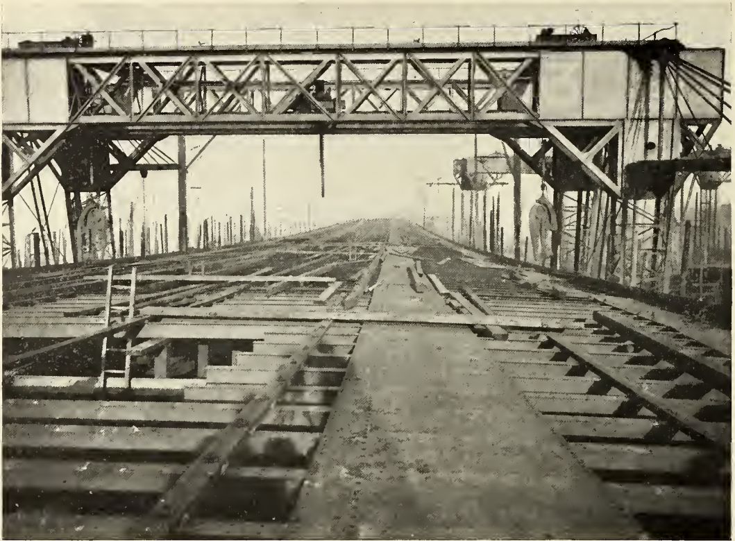
THIS IS NOT A RAILROAD BUT MERELY THE PROMENADE DECK OF THE ADRIATIC IN COURSE OF CONSTRUCTION AT BELFAST.
