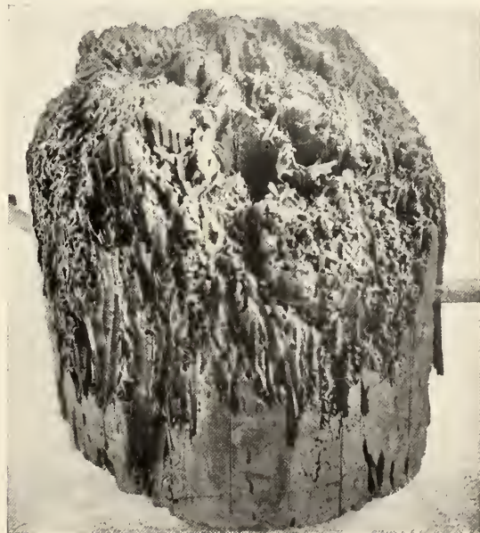
WHARF PILE BORED BY A TEREDO.
