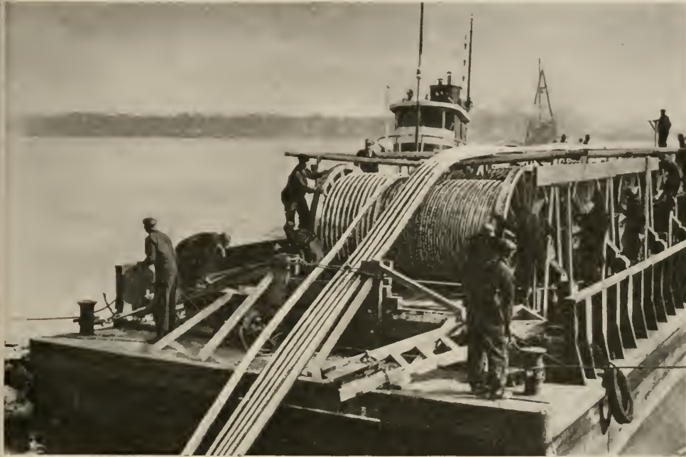
CABLES UNDER THE POTOMAC
