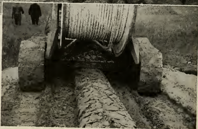
FIG. 33. Back-filling is part of the cable-laying operation. A device under the rear trailer mounds up the earth over the furrow, and a tractor runs over it when bringing up a new reel of cable
