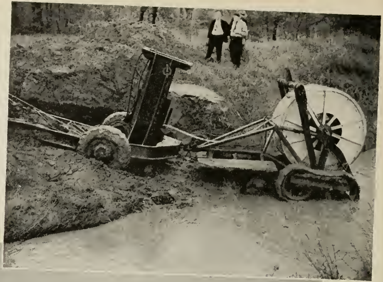
FIG. 10, right: A bulldozer has already opened up a passage for the plow train in the bank of this creek. FIG. 11, below: Crossing a road at an angle often obviates cutting away shoulders or banks
