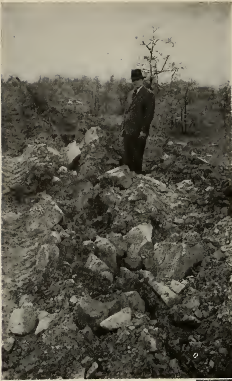
FIG. 3, left: Where ground conditions are as bad as this, the rooter plow goes ahead, and the cable-laying plow follows as a separate operation. FIG. 4, below: Power applied from the single-drum winch of a stationary tractor comes in handy for pulling the train, or any part of it, up hills or out of mud
