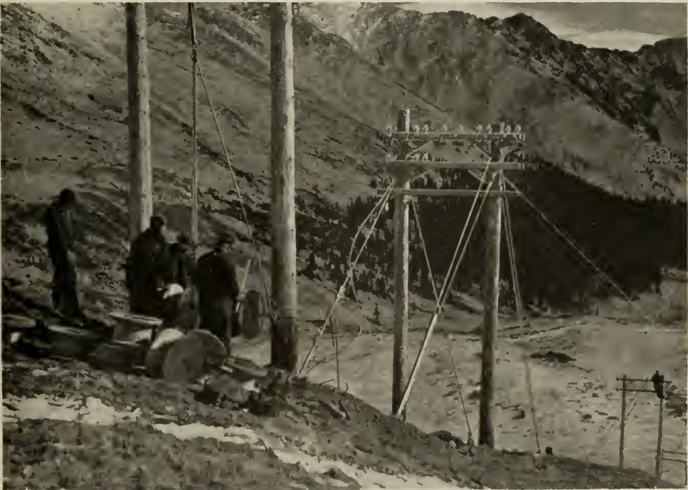
CONSTRUCTION NEAR THE SUMMIT The crew is preparing to string the stranded copper conductors. Note the heavy construction and guying shown on the H-structure in the center of this picture
