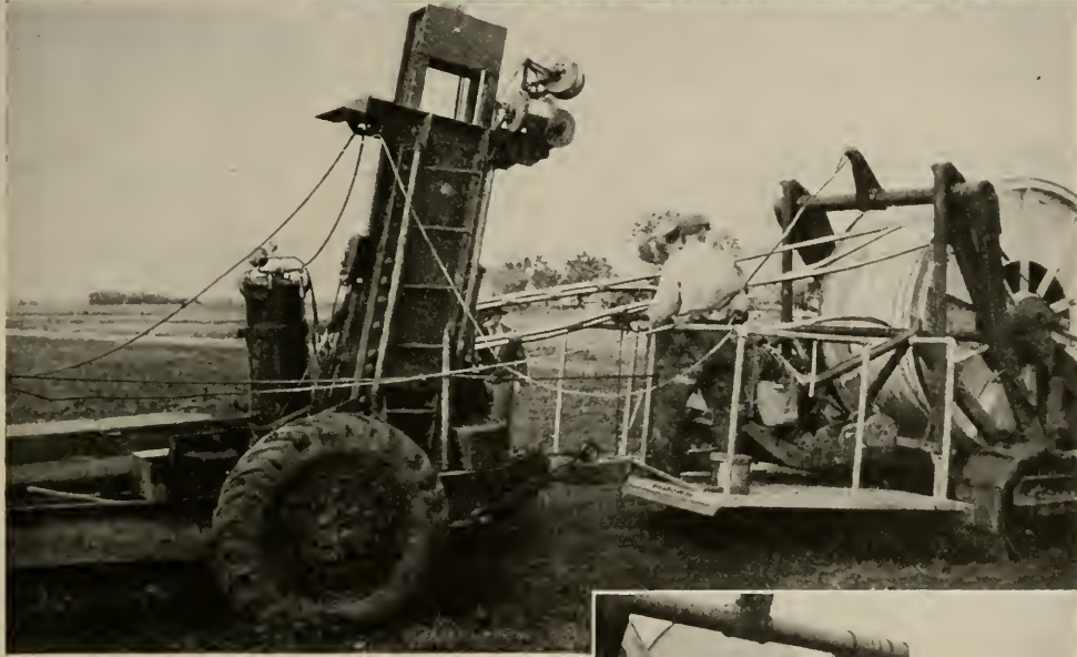
FIG. 27. Guiding clamped cables into the plow share. Cables must enter the share in proper position to obviate binding
