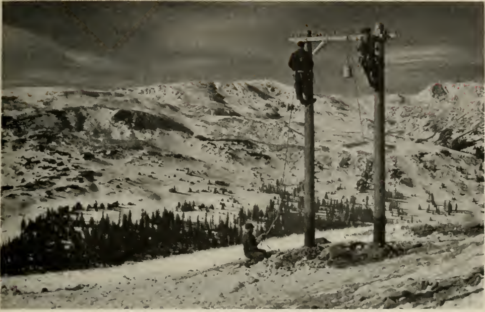
GRANDSTAND VIEW Construction of an H-structure on the crest of Loveland Pass
