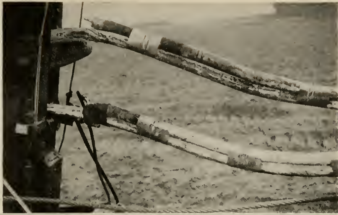
FIG. 26. Each succeeding cable is clamped to the end of the cable ahead, in order to pull it into the plow share
