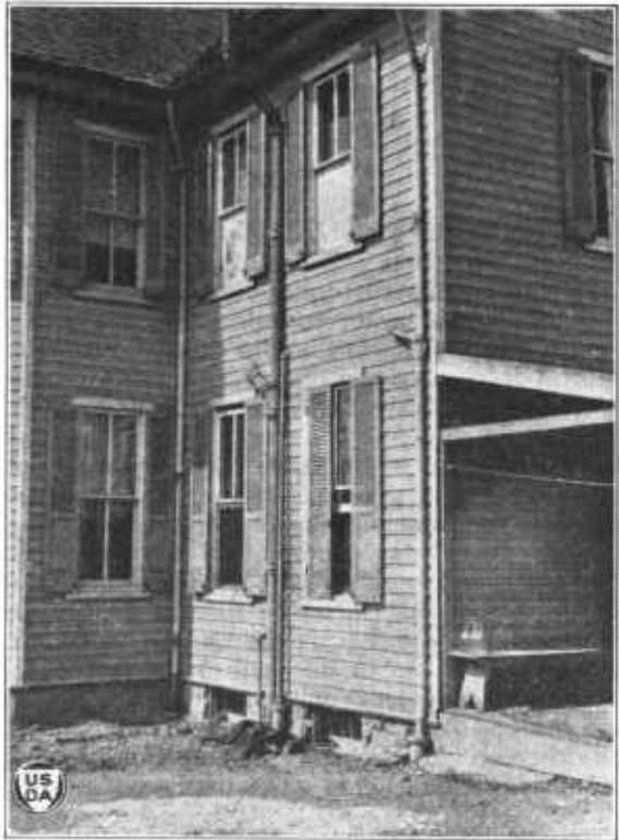
FIG. 2.—Home plumbing in Maryland, installed by one man unaided; no trouble from frost in 15 years because the faucets do not drip; the soil and vent stack is at the center of the ell; the sink waste is low and just to the left; the washstand waste is just to the right of the soil stack; the bathtub waste enters the rain conductor at the near corner and immediately above the porch roof. Outside soil stacks are unsightly but are often installed in mild and moderate climates such as in southern United States and in England
