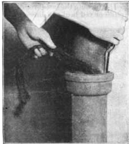
FIG. 10.—Use of a yarning iron to pack a strand of oakum or jute into the bottom of the joint space
