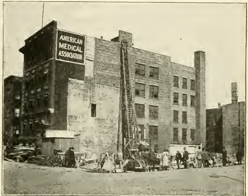
Fig. 8.—General view of the excavation and the old building, with the pile-driver in place.
