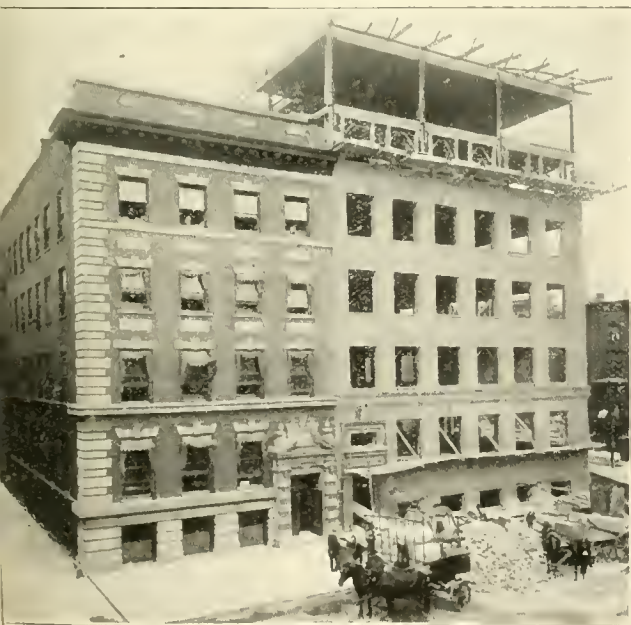
Fig. 14.—View of the fronts of the old and new buildings, the brick work of the latter nearing completion.
