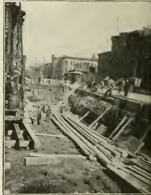
Fig. 6.—Another view of the excavation with the pile-driver at the left and some of the 50-foot piles. Holes in the ground show where piles have already been driven.
