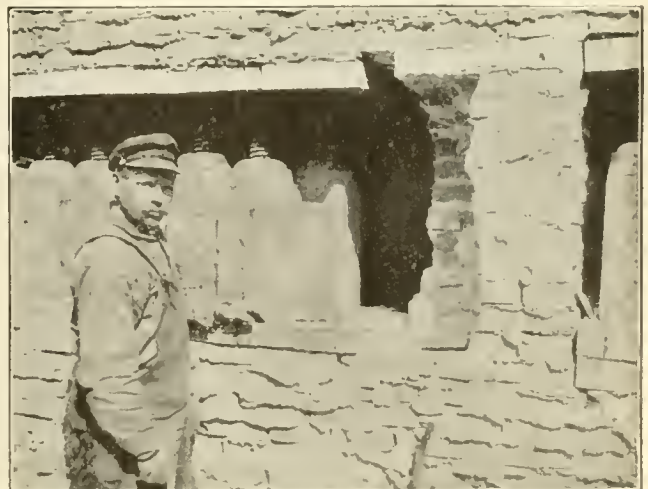
Fig. 9.—Wall of the old building, showing the method of preventing collapse or damage to the building by the driving of the piles.
