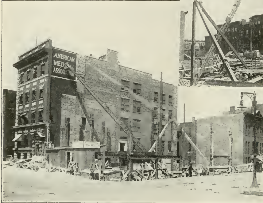
Figs. 10 and 11.—The steel skeleton of the building as it appeared after the first few beams were erected. The small picture shows another view of the electric crane which handled the heavy beams; as each one was swung into place it was temporarily secured by bolts and nuts. These were later replaced by rivets placed while hot and securely riveted by compressed-air machines.
