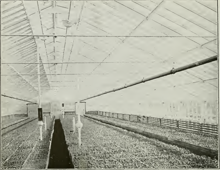
Double ridge ventilation and side ventilators on both sides are found in this house. Ridge ventilators operated in centre of house by two gear supports.
