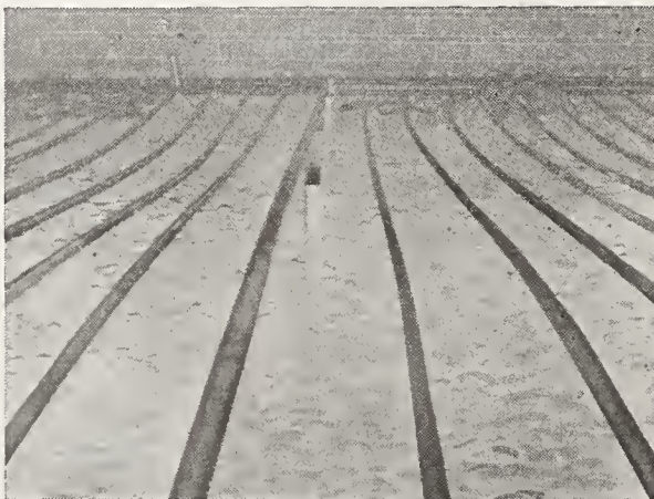
Pipe grid coils which heat floor of the Jewell Valley theatre, shown before laying of concrete slab.
