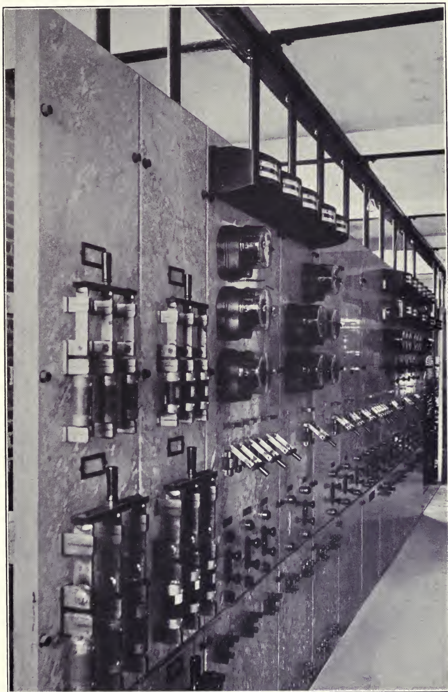
SWITCHBOARD, WASHINGTON STREET STATION
