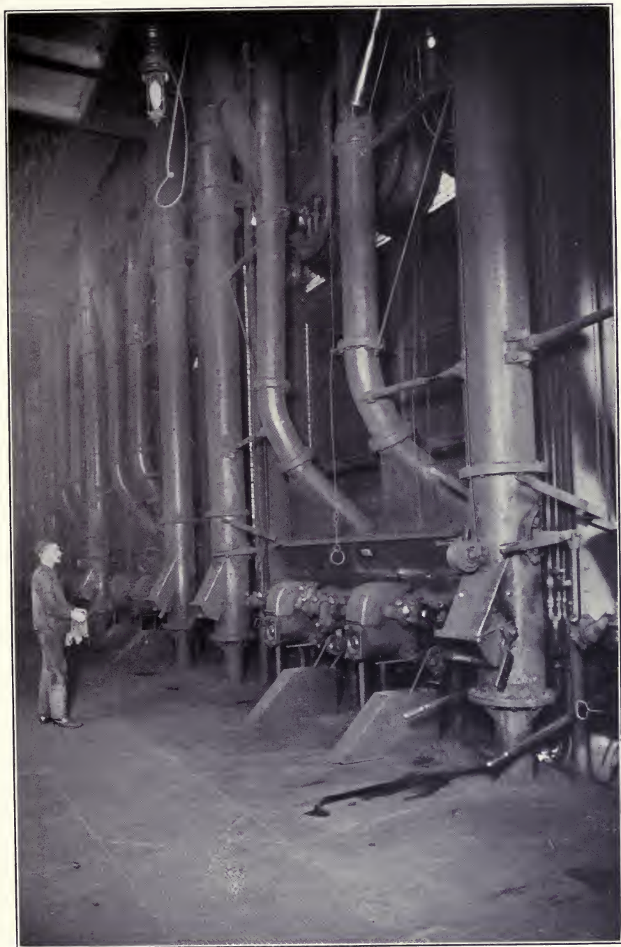
FIRING AISLE, WATERSIDE STATION NO. 2
