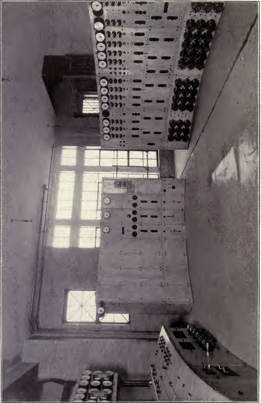
HIGH TENSION SWITCHBOARD, MILLERS FORD STATION.
