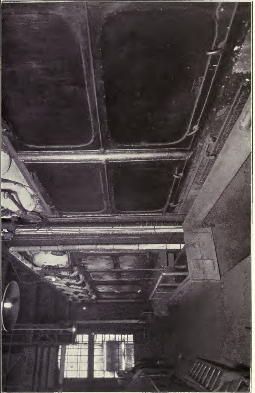
FIRING AISLE, PRUDENTIAL OIL CORPORATION
