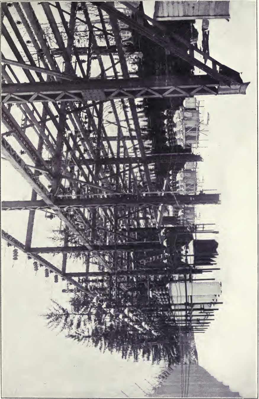
SUBSTATION, TRENTON FALLS, UTICA GAS AND ELECTRIC CO.
