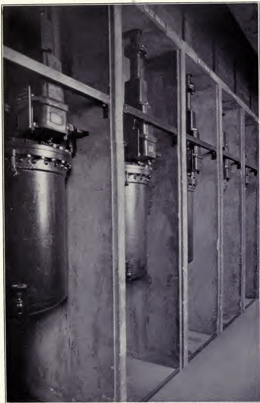
FEEDEE SWITCHES, HELL GATE STATION
