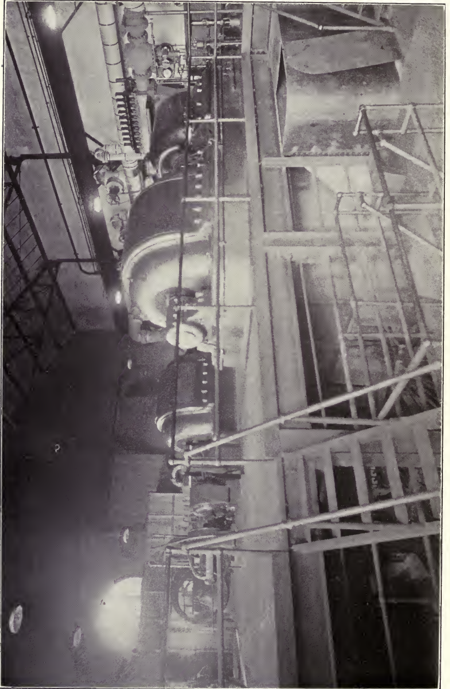
TURBINE ROOM, WASHINGTON STREET STATION
