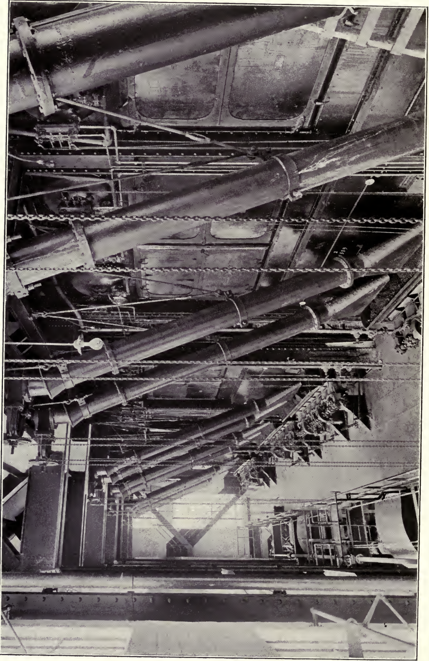
FIRING AISLE, RIVERSIDE STATION
