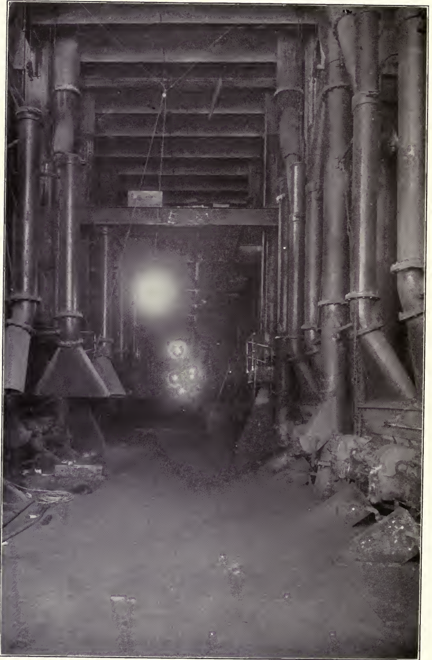
FIRING AISLE, SHERMAN CREEK STATION
