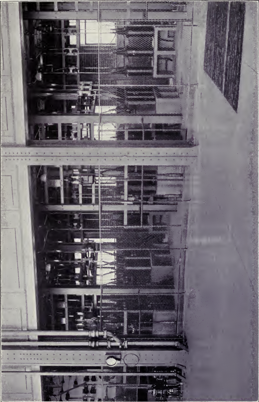
12,000-VOLT SWITCHING EQUIPMENT, COHOES STATION
