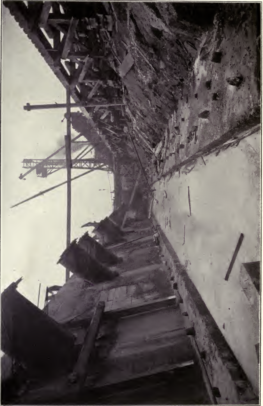
INSIDE OF SEA WALL AND BOTTOM OF DISCHARGE TUNNEL, HELL GATE STATION
