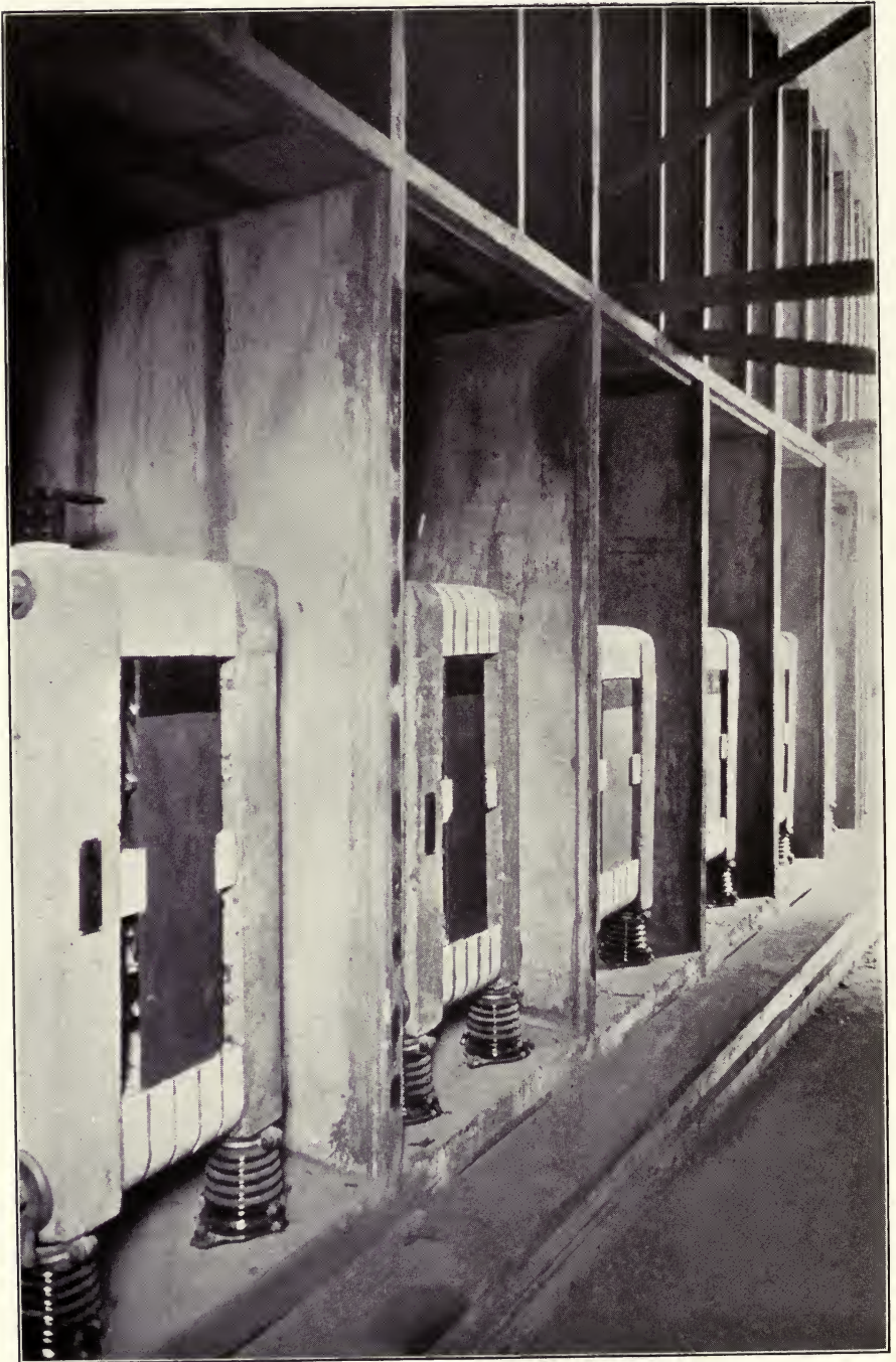
REACTANCE COILS, HELL GATE STATION
