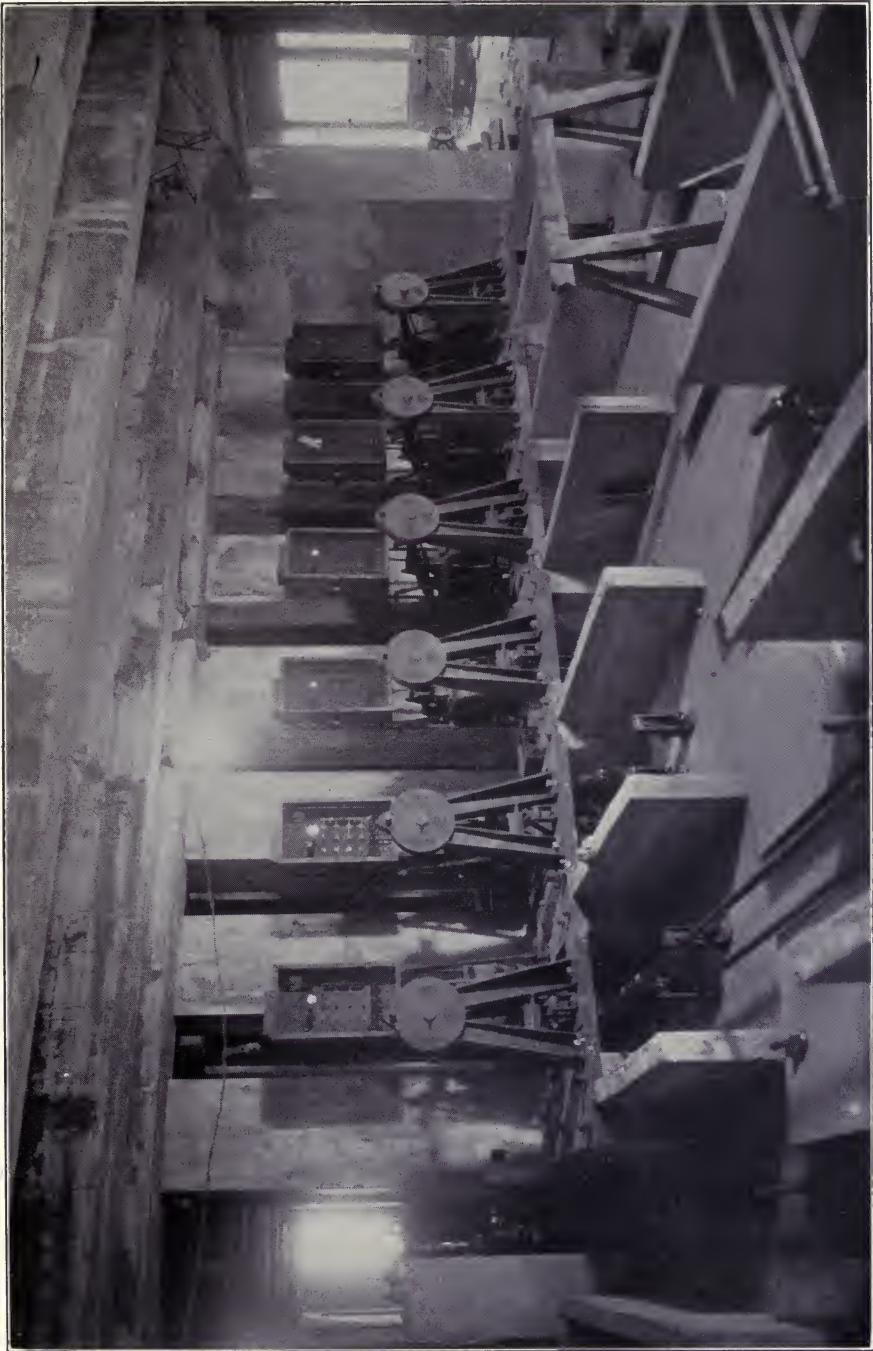
OPERATING MECHANISM FOR SWITCHES, HELL GATE STATION
