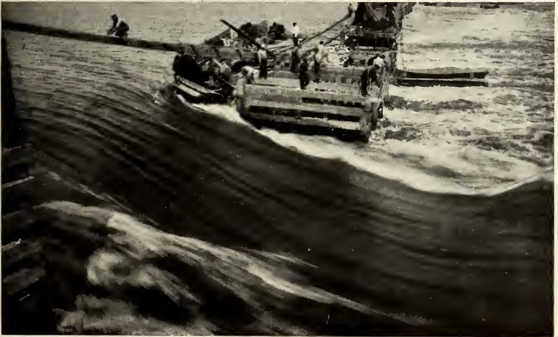
THE FINAL STRUGGLE OF THE RIVER AS THE LAST GAP WAS BEING CLOSED.
