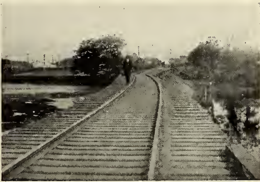
THE RAILROAD TRACK THAT SLIPPED.
