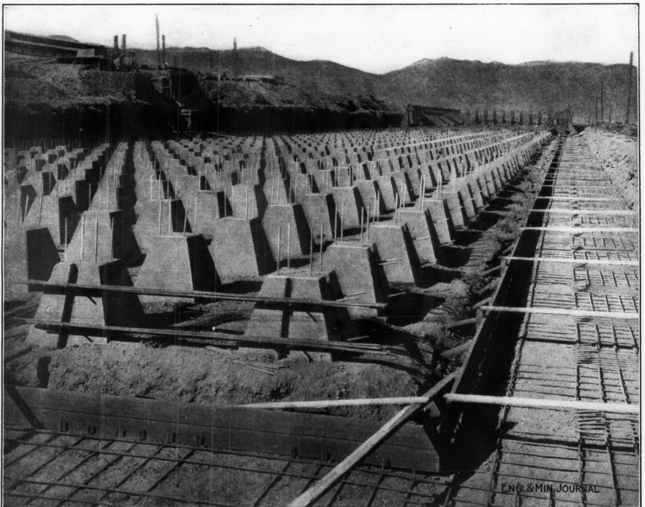
FOOTINGS FOR LEACHING VATS NOS. 5 AND 6, FORMS FOR NORTH, EAST AND SOUTH WALLS IN REAR
