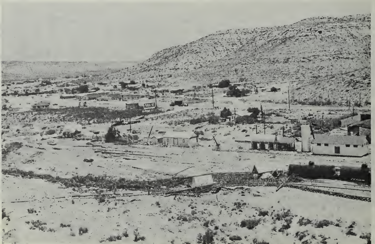
Aerial view, looking northwest, showing damages to Southern Pacific railroad. Note workmen repairing railroad bridge in left of photo.
