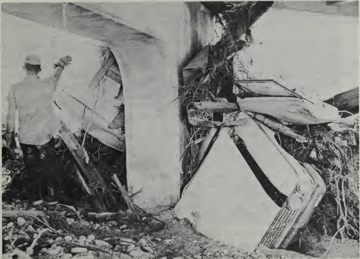
Automobile swept downstream against bridge support.
